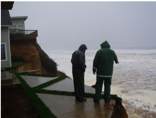
Figure 2-37. Bluff Failure Due to Toe Erosion by Ocean Waves
