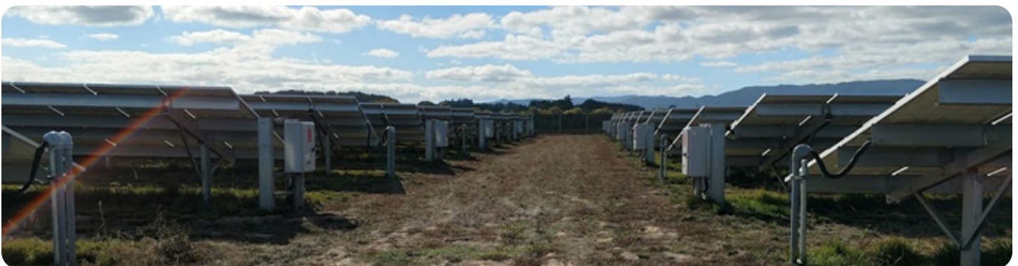
Oregon Solar Farm, Willamette Valley
