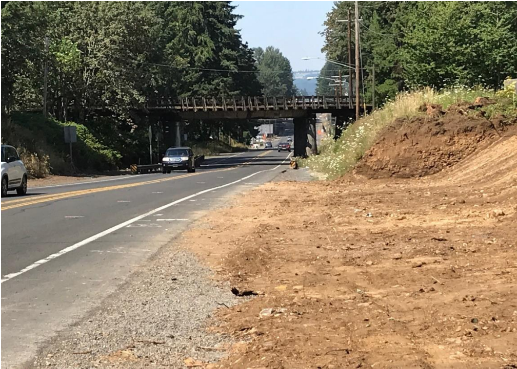
New curb and sidewalk will be constructed from 55 th Ave to 60 th Ave
