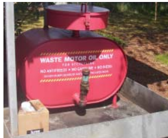
Waste oil tank at Tomahawk Bay Marina
