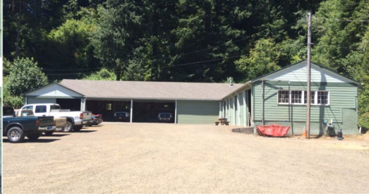
Northwest corner on Truck/Automotive Shop -Shows hillside encroaching on building -Shows old brick and mortar foundation
