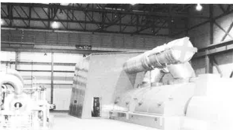
Left: one of the huge generators. To gain an idea of the scale: the door to the left of the generator is standard size.
