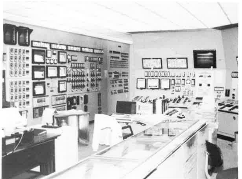
Above: the control room is much the same as would be seen in other modern power-producing facilities.
