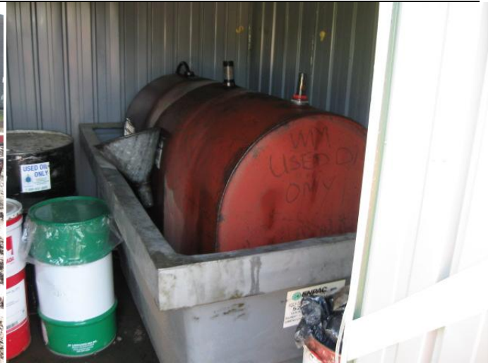
Used oil container. This is used by the facility. When customers bring in used oil, which is rare, it is placed in this tank.
