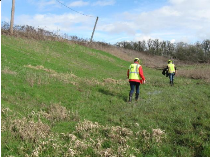
Southern perimeter berm (1 of 4). Following recent flooding of the area south of the landfill, the berm was inspected for signs of scouring or erosion. The berm appears to be in good condition.
