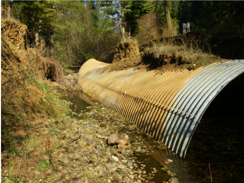
Figure 3-8. Washed out culvert on East Pine Creek approximately 5 miles north of Halfway, OR. Recent floods have caused similar damage throughout the Pine Valley. (DEQ 2010)
