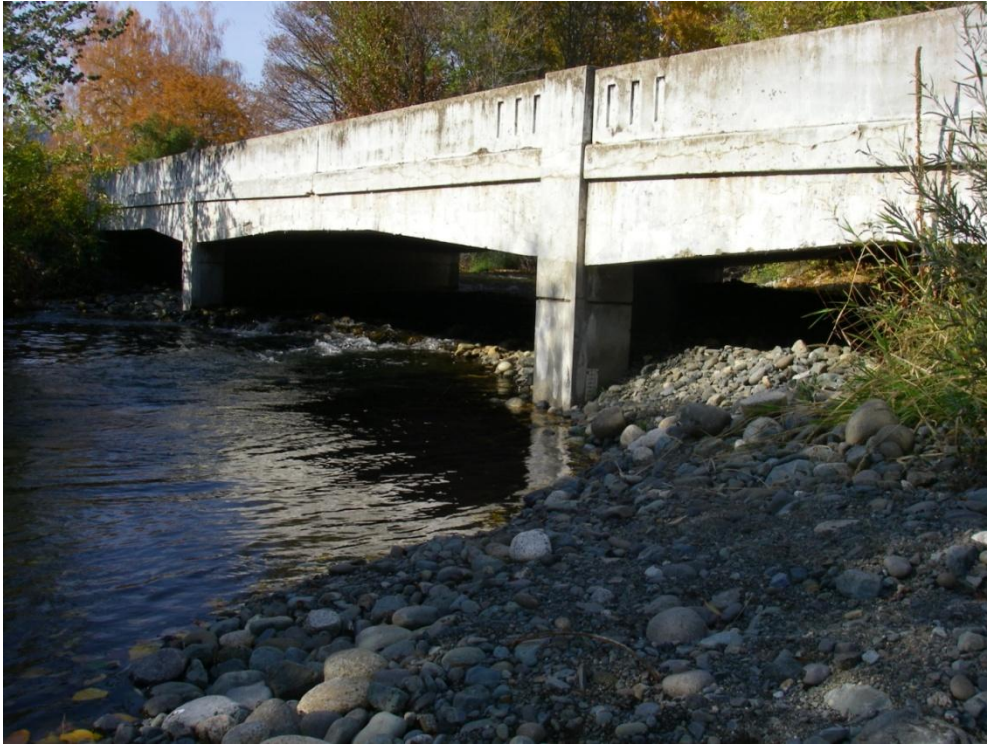
Figure 3-7. Highway 414 bridge located immediately upstream of the City of Halfway wastewater treatment plant. Channel under the bridge has filled with gravel and cobble stream sediment leaving only a few feet of space for passing flows in Pine Creek. (DEQ, 2010)
