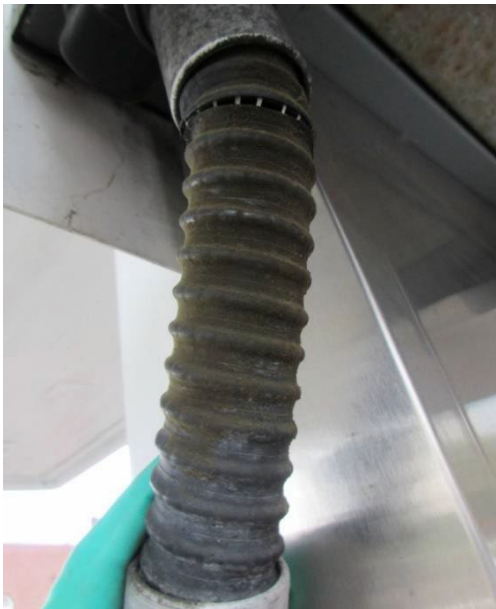
(AQGP-23) Balance whip hose- torn
