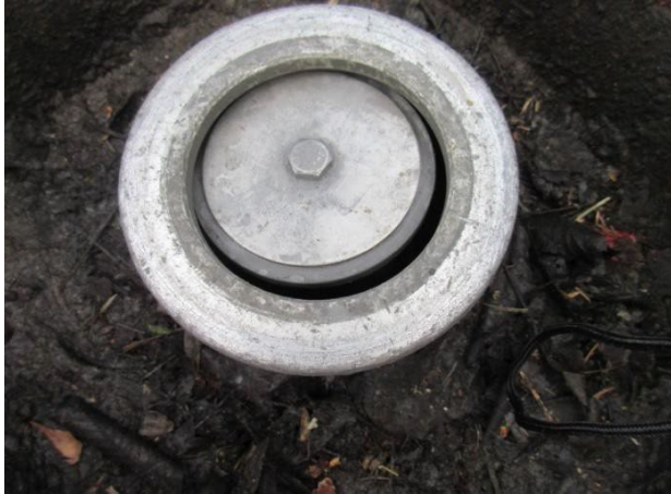
(AQGP-22 & 23) Poppet valve not sealing.
