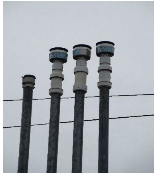
(AQGP-22 & 23) This picture shows three PV valves, one for each gasoline tank on site, and one open atmospheric vent (left) piped to the diesel tank. Note that one PV valve is acceptable for multiple gasoline tanks if the piping is manifolded together. All Stage II permitted sites require PV valves for gasoline storage tanks. Refer to your permit to determine whether this is required at your site.
