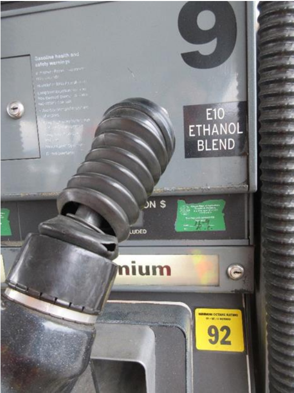
Balance System- bellows torn
