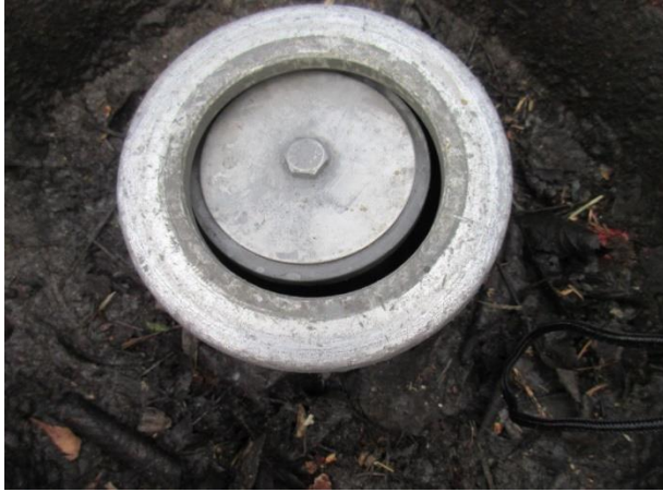
Poppet valve not sealing.
