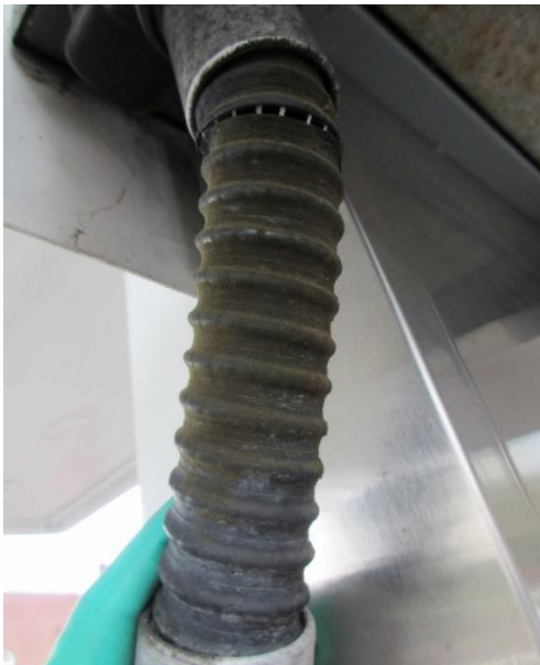
Balance whip hose- torn
