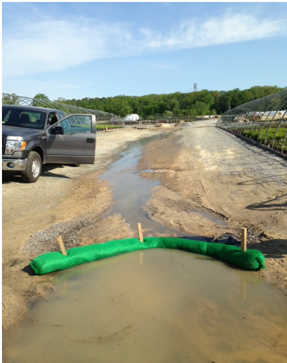
Image 4. Ponding effect behind filter sock.
