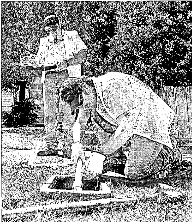
Creighton Nevin, front, and Joe Watson of the Medford Water Commission check meters Monday for galvanized pipe on West Eighth Street. MAIL TRIBUNE / DENISE BARATTA
