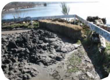
Poorly Confined Spoils
