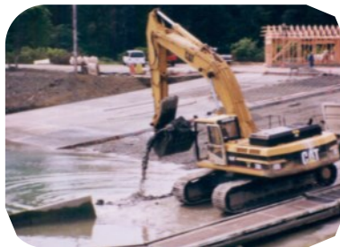
Poor Bucket Control
