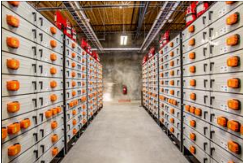
The PGE Smart Power project is 5 MW of battery storage, primarily for renewable energy power output firming and shaping.
