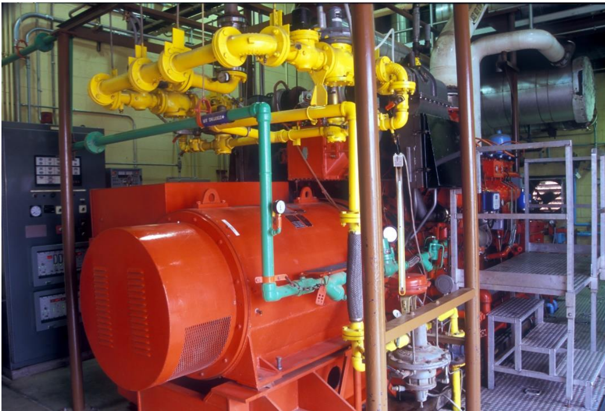
The Willow Lakes cogeneration facility.
