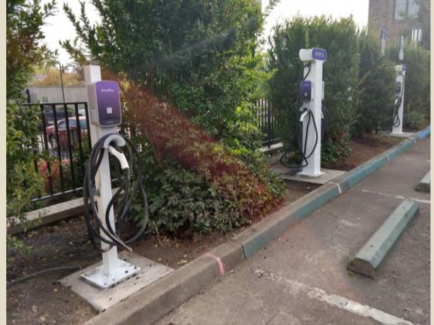
In 2020, the City of Ashland installed free public EV chargers using Oregon Clean Fuels Program credits.
