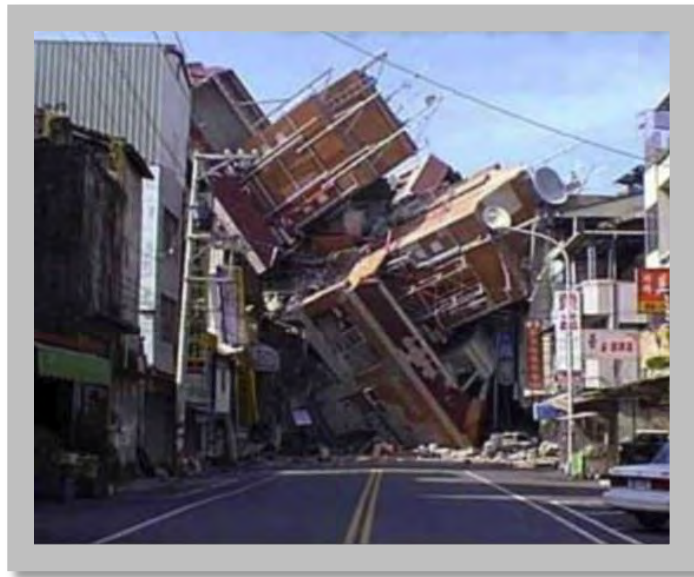
Figure 7.10: Cell site collapsed with the commercial building collapse. Chi Chi earthquake, Taiwan, 1999. (Source: Alex Tang)
