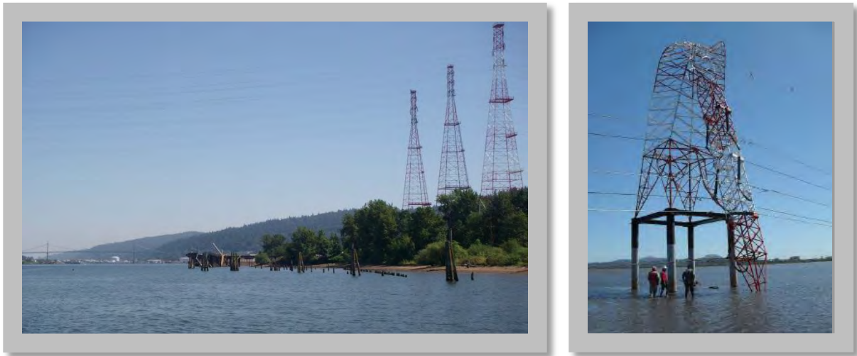
Left: These high voltage electrical transmission towers are built on a river bank in the Critical Energy Infrastructure (CEI) Hub susceptible to lateral spreading. (DOGAMI photo) Right: Structural damage to a high voltage transmission tower located at a river crossing in 2010 Chile earthquake (ASCE Technical Council on Lifeline Earthquake Engineering – TCLEE)
