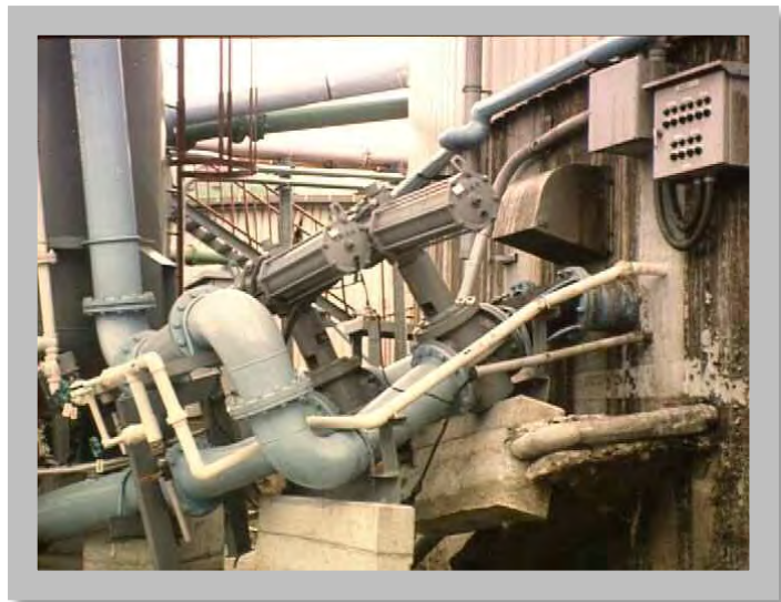
Figure 8.15: Damage from liquefaction/lateral spreading at Higashinada WWTP, Kobe, Japan, 1995 (Source: Photo by Don Ballantyne)
