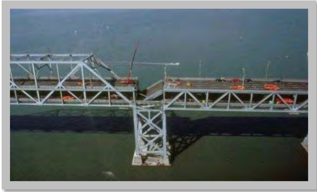
Figure 7.1: San Francisco – Oakland Bay Bridge after the 1989 Loma Prieta earthquake. An example of bridge failures that could impact utility conduits supported by or integrated into the bridge. Source: U.S. Department of Transportation. (Source: USGS website http://earthquake.usgs.gov/earthquakes/states/events/1989_10_18.php )
