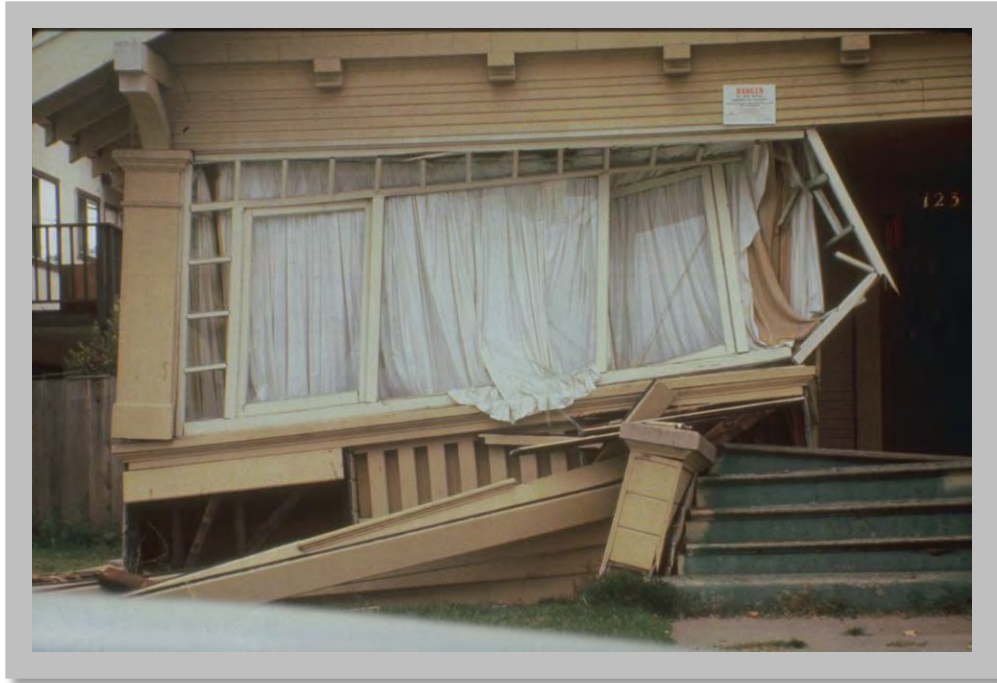
Figure 4.8: This residential building shifted on its foundation after the 1989 M 7.1 Loma Prieta, California earthquake. (Source: NOAA/NGDC, C. Stover, U.S. Geological Survey)
