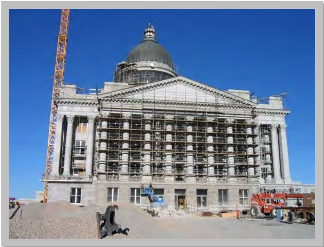
Figure 4.7: Several states have rehabilitated their state capitol buildings. The Utah State Capitol was seismically retrofitted with base isolation to protect visitors and occupants and preserve historic fabric in the building. (Source: State of Utah)
