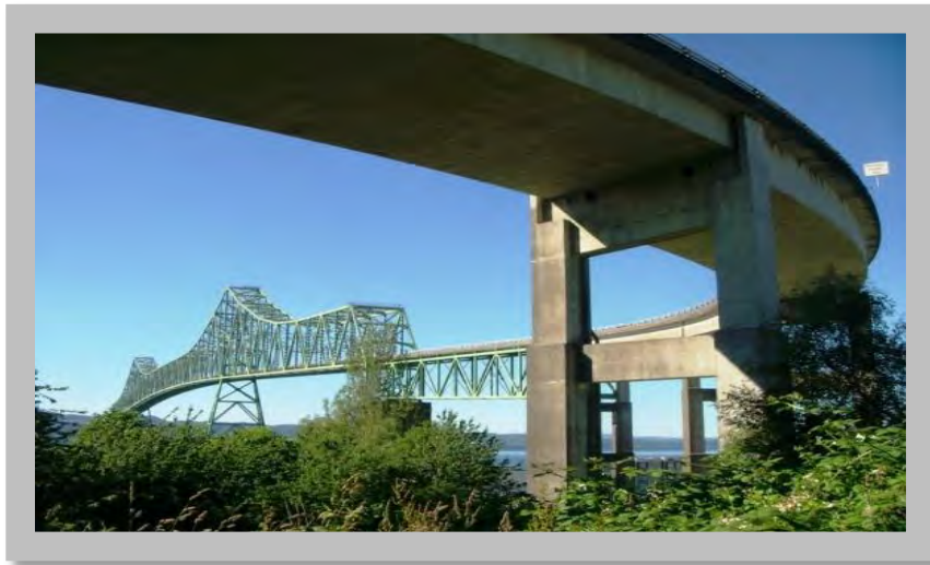
The approach (foreground) to the 1966 Astoria-Megler Bridge that spans the Columbia River has major structural deficiencies that could lead to a collapse following an earthquake. Damaged bridge sections could block waterway access to the Critical Energy Infrastructure Hub. (DOGAMI photo)
