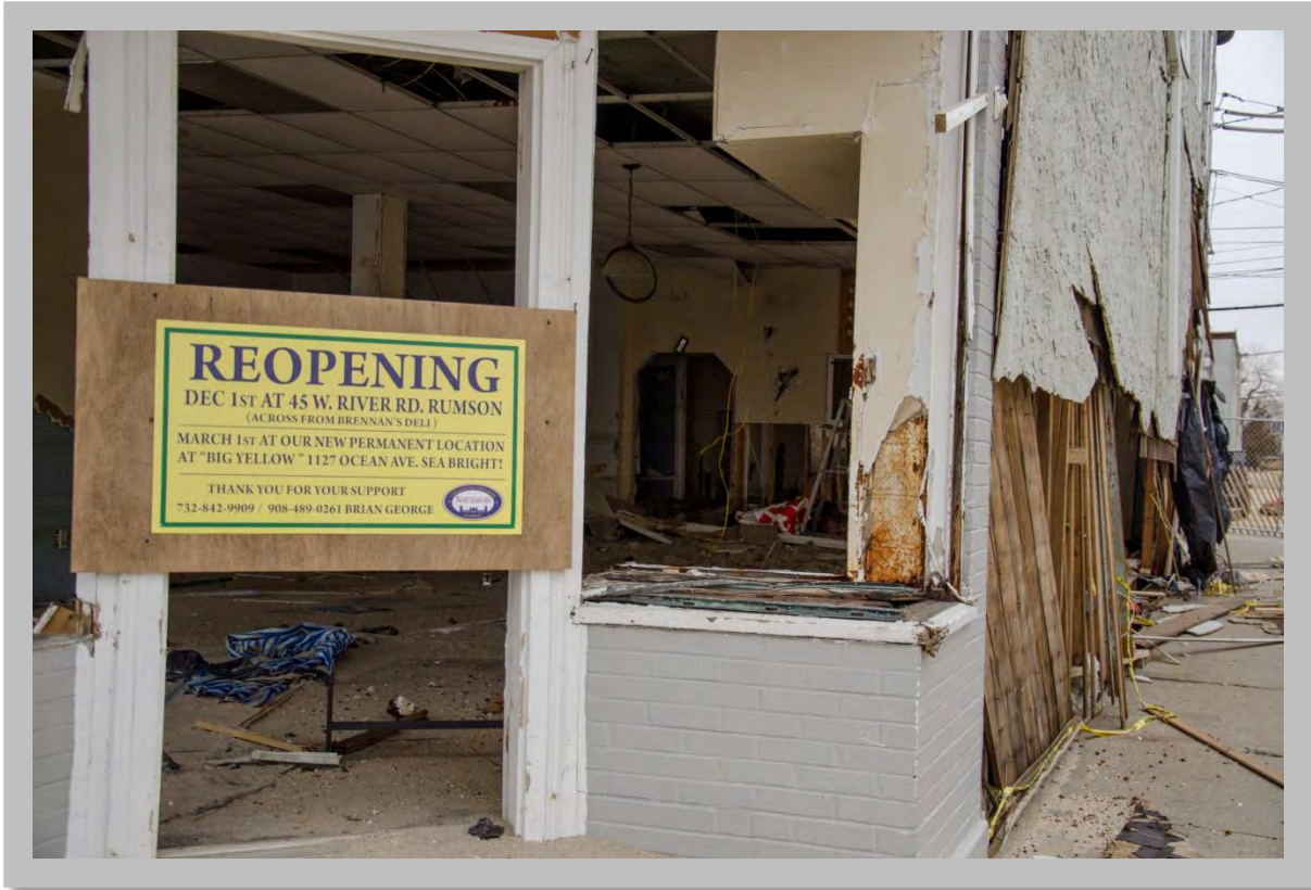
Figure 2.10: Sea Bright, N.J., Jan. 25, 2013 -- Some businesses have permanently relocated to higher ground after being destroyed by Hurricane Sandy. (Source: Photo by Liz Roll/FEMA)
