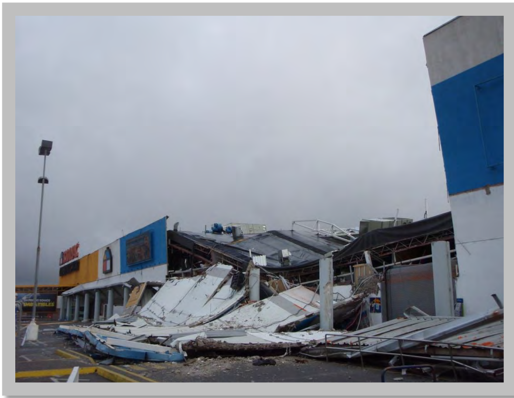
Figure 4.9: Several tilt-up concrete panels of this construction material supply store in Concepcion fell away from the building, causing the roof framing to collapse after the M 8.8 February 27, 2010 Maule Chile earthquake. (Source: Kent Yu, Degenkolb Engineers)
