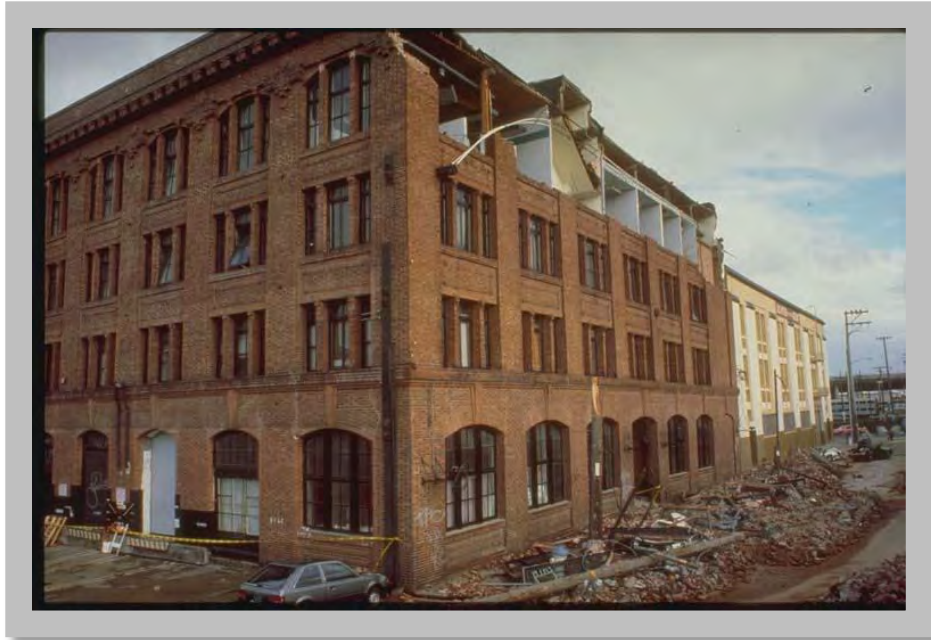
Figure 4.11: The fourth-story wall of this unreinforced masonry building on Bluxome Street in San Francisco collapsed onto the street, killing five people in their cars, during the M7.1 October 18, 1989 Loma Prieta, California earthquake. (Source: NOAA/NGDC, E.V. Leyendecker, U.S. Geological Survey)
