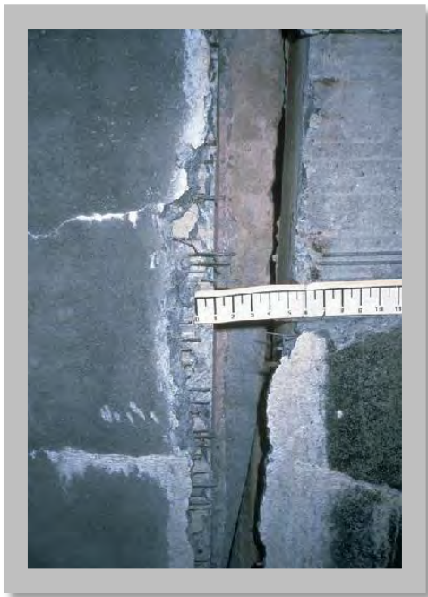
Figure 8.3: Wire wrapped concrete tank burst in Purisima Hills, Loma Prieta earthquake, California, 1989 (Source: Photo by Don Ballantyne)
