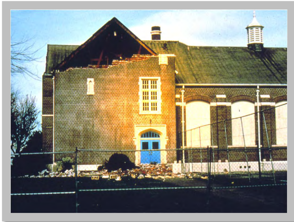
Figure 4.5: The previous Molalla High School building, a three-story unreinforced masonry structure, was damaged from the M5 .6 Scotts Mills, Oregon earthquake in 1993. It happened during spring break, when the school was empty, which prevented serious injuries. The district took the opportunity to forecast future needs and decided not to rebuild at the same location. Molalla High School is now housed on a larger campus with a stronger, more spacious building. Many URM schools and other buildings in Oregon could suffer a similar fate in future earthquakes. Communities can act now to plan how and when to rehabilitate or replace these aging, potentially dangerous facilities. (Source: DOGAMI)
