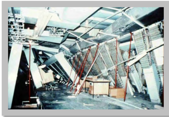
Figure 7.9: Inadequate anchorage and poor overhead bracing details resulted in equipment toppling. Mexico City earthquake, 1985. (Source: Alex Tang)
