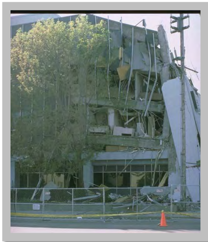
Figure 4.12: This non-ductile concrete frame medical building collapsed during the 1994 M6.8 Northridge, California earthquake. (Source: NOAA/NGDC, J. Dewey, U.S. Geological Survey)
