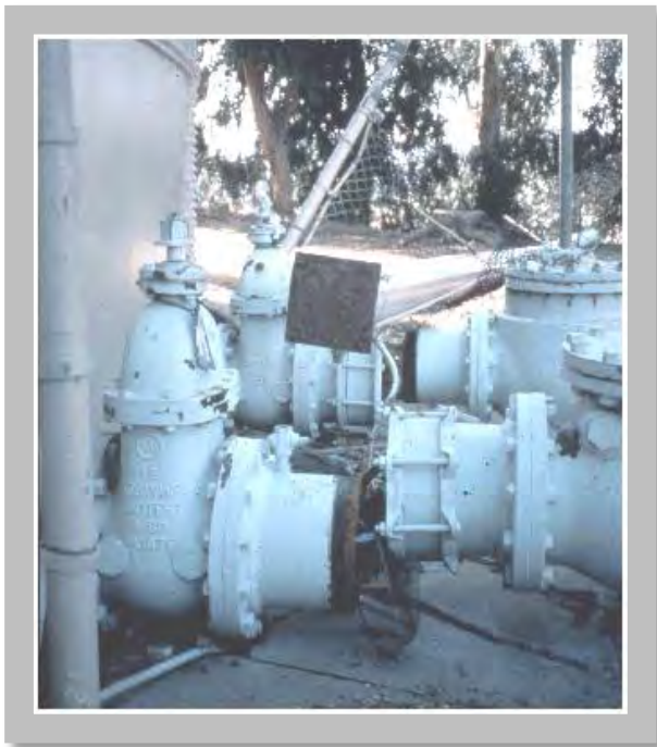
Figure 8.1: Tank piping separated, Northridge earthquake, California, 1994 (Source: Los Angeles Department of Water and Power)
