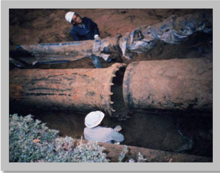
Figure 8.5: Pipelines separated, Great Hanshin earthquake, Kobe, Japan, 1995 (Source: Kobe Water Department)
