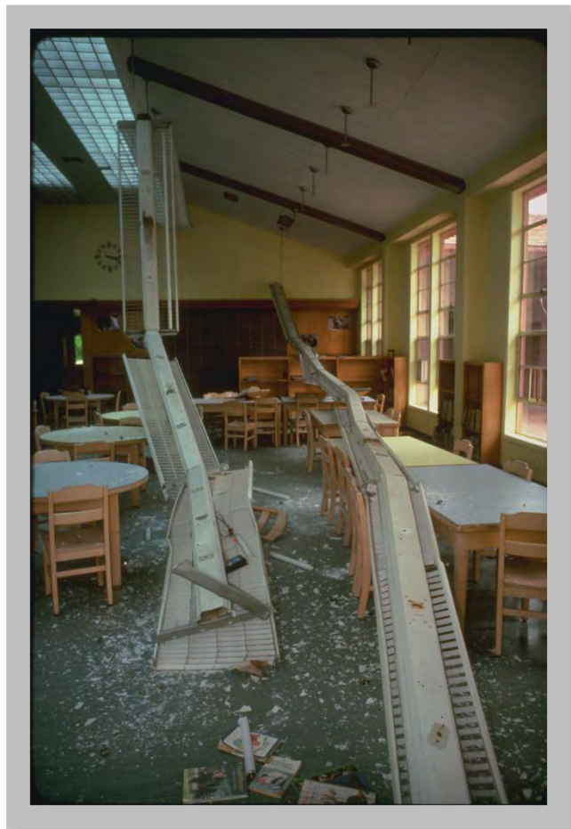
Figure 4.6: Pendant light fixtures failed in this elementary school library during the 1983 M6.5 Coalinga, California earthquake. If the room had been occupied, this could have caused injuries. Bracing nonstructural elements in homes, schools, and offices can often be done easily and relatively inexpensively. (Source: NOAA/NGDC, Earthquake Engineering Research Institute)
