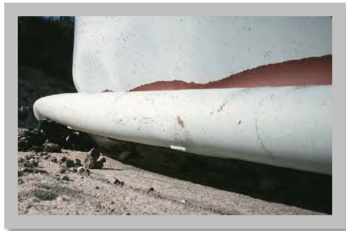
Figure 8.2: Tank buckling, Northridge earthquake, California, 1994 (Source: Photo by Don Ballantyne)
