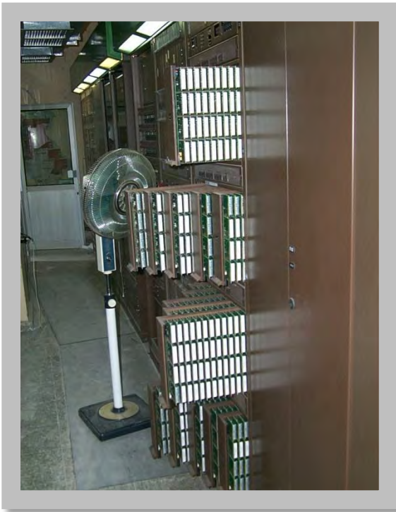
Figure 7.8: Circuit Boards pulled out and fan to get some air cooling due to failure of the air conditioning unit. Fortunately, the site had power and they could open windows to allow cool air to come in. Izmit (Kocaeli) earthquake, Turkey, 1999. (Source: Alex Tang)
