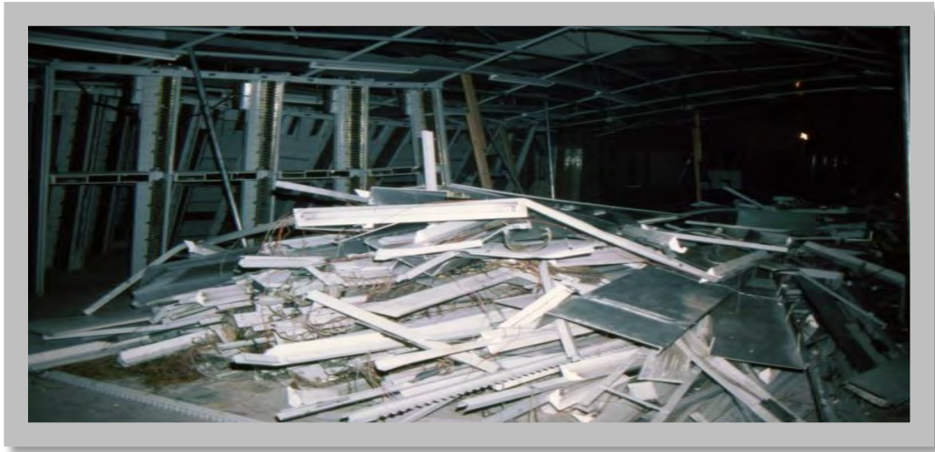
Figure 7.2: The overhead lighting fixtures in a Central Office failed during an earthquake. Note the equipment in the background was supported by “jiffy poles” after the earthquake. Mexico City earthquake, 1985. (Source: Alex Tang)
