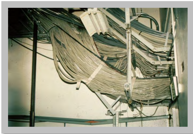
Figure 7.3: Overloaded cable rack failed in relatively minor (M=5.8), Whittier Narrows earthquake, California, 1987. (Source: Alex Tang)
