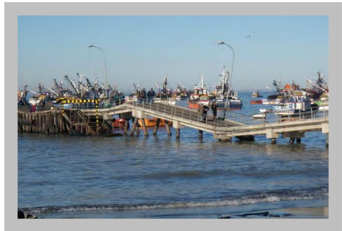
Figure 6.6: An example of a damaged pier in the 2010 Chile earthquake (ASCE Technical Council on Lifeline Earthquake Engineering – TCLEE, 2010)
