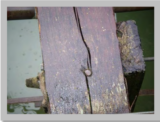
Figure 6.9: The connection on this pier in the CEI Hub appears to have deteriorated due to a split in the timber beam. This type of damage suggests that the condition of the structure may not be routinely monitored and maintained and that the overall pier is seismically vulnerable (Source: DOGAMI photo)
