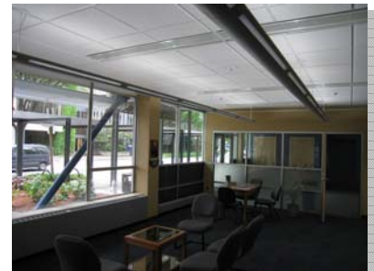
Chilled beams and indirect lighting highlight the innovative energy conservation measures incorporated into the Eugene State Office Building
