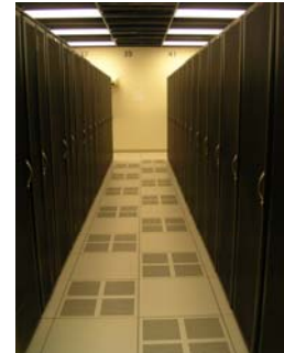
Hot and cold server rows at Oregon's State Data Center
