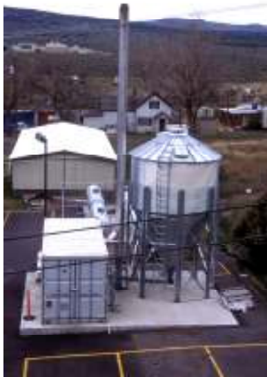
Biomass heating facility at the Harney Hospital in Burns, OR
