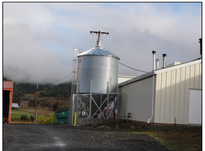
Days Creek Charter School installed a new biomass boiler to replace an inefficient and costly donated oil-fired boiler. The biomass boiler was paid for in part with Recovery Act (stimulus) funds from the Oregon Department of Energy
