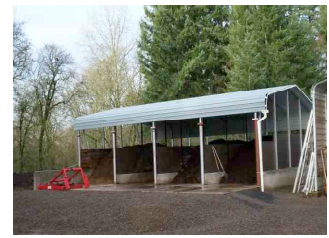
Potential solutions: covered manure storage/compost facility
