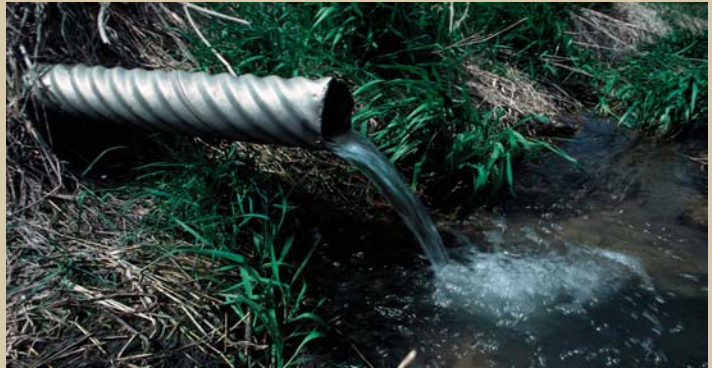
Tile outlets that run during the irrigation season are indicators of over watering.
