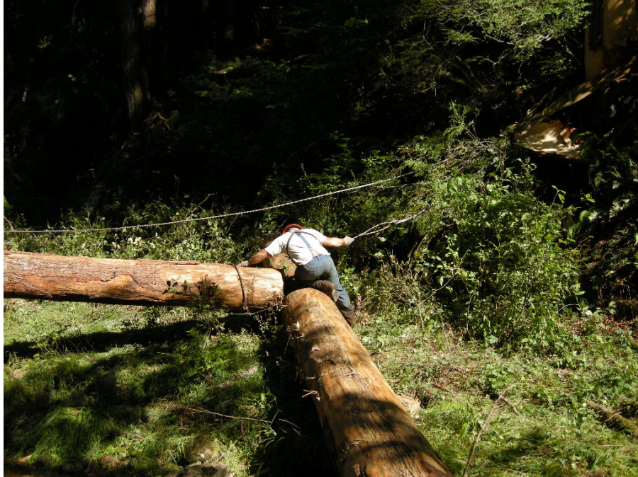
Hooking up cables to pull wood into the stream channel on Elk Creek.
