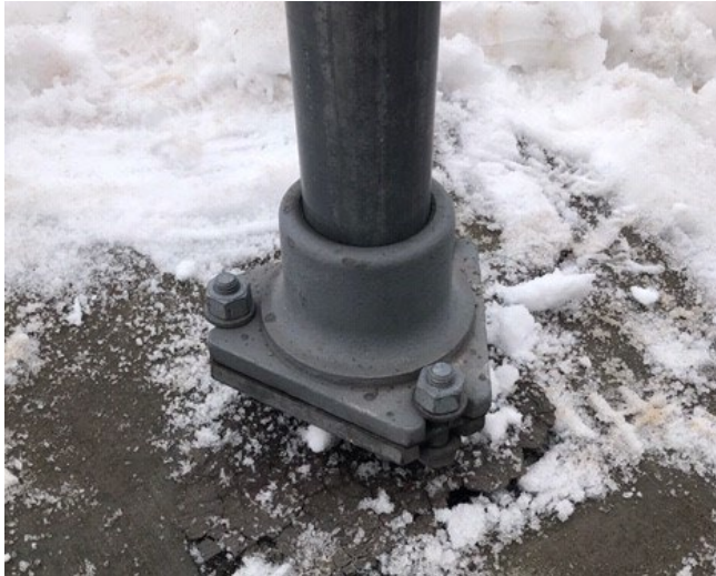
Figure 4: Triangular base breakaway with a round post; a standard no longer supported by ODOT.
