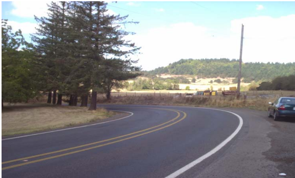
Photograph No. 2 — Substandard curve, north of
