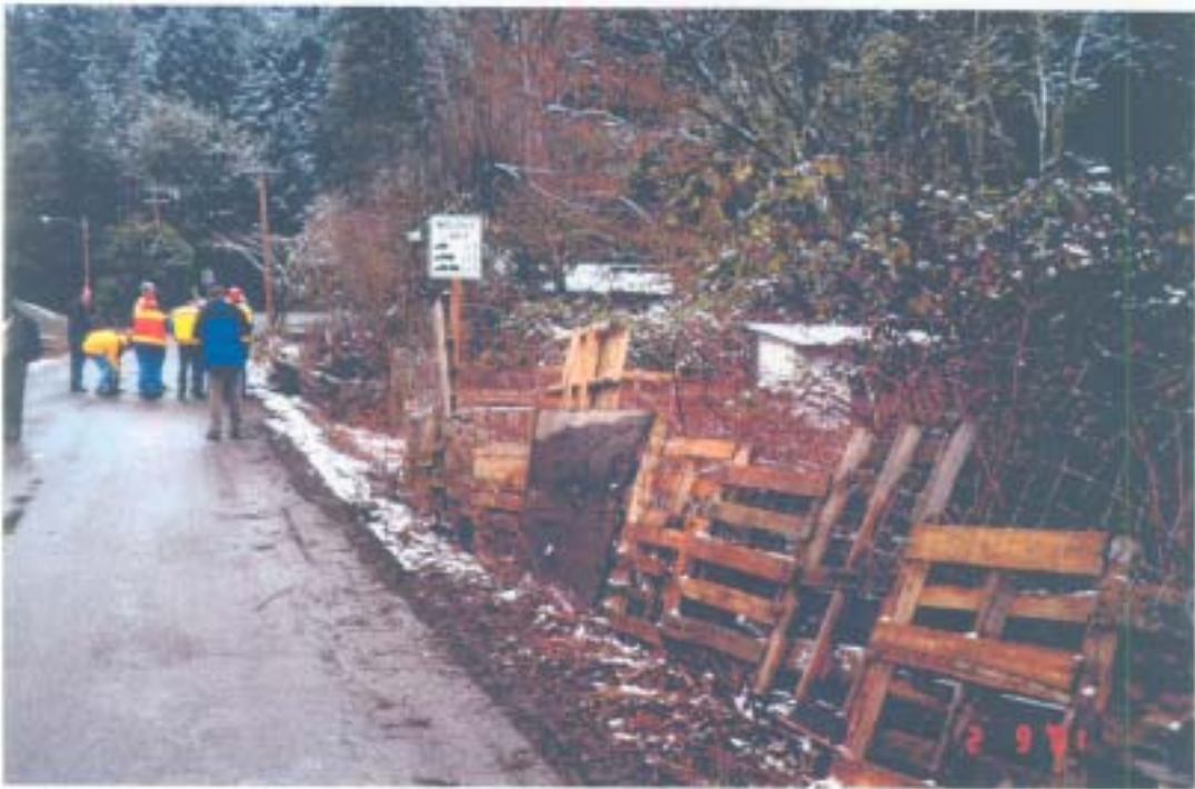
Looking north at the bridge from the south approach. Fence along east side.
