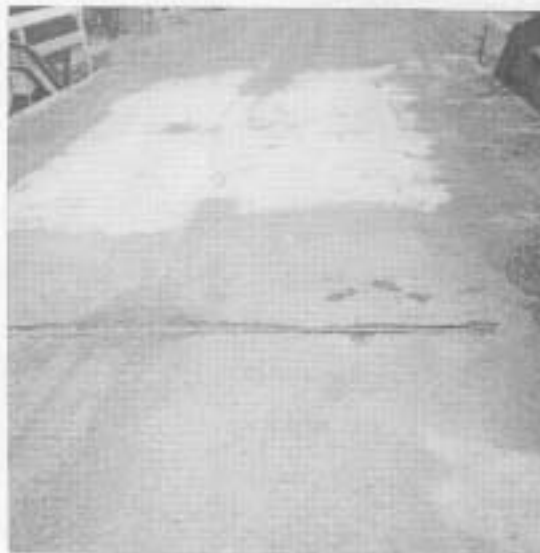
exposed rebar top of deck
