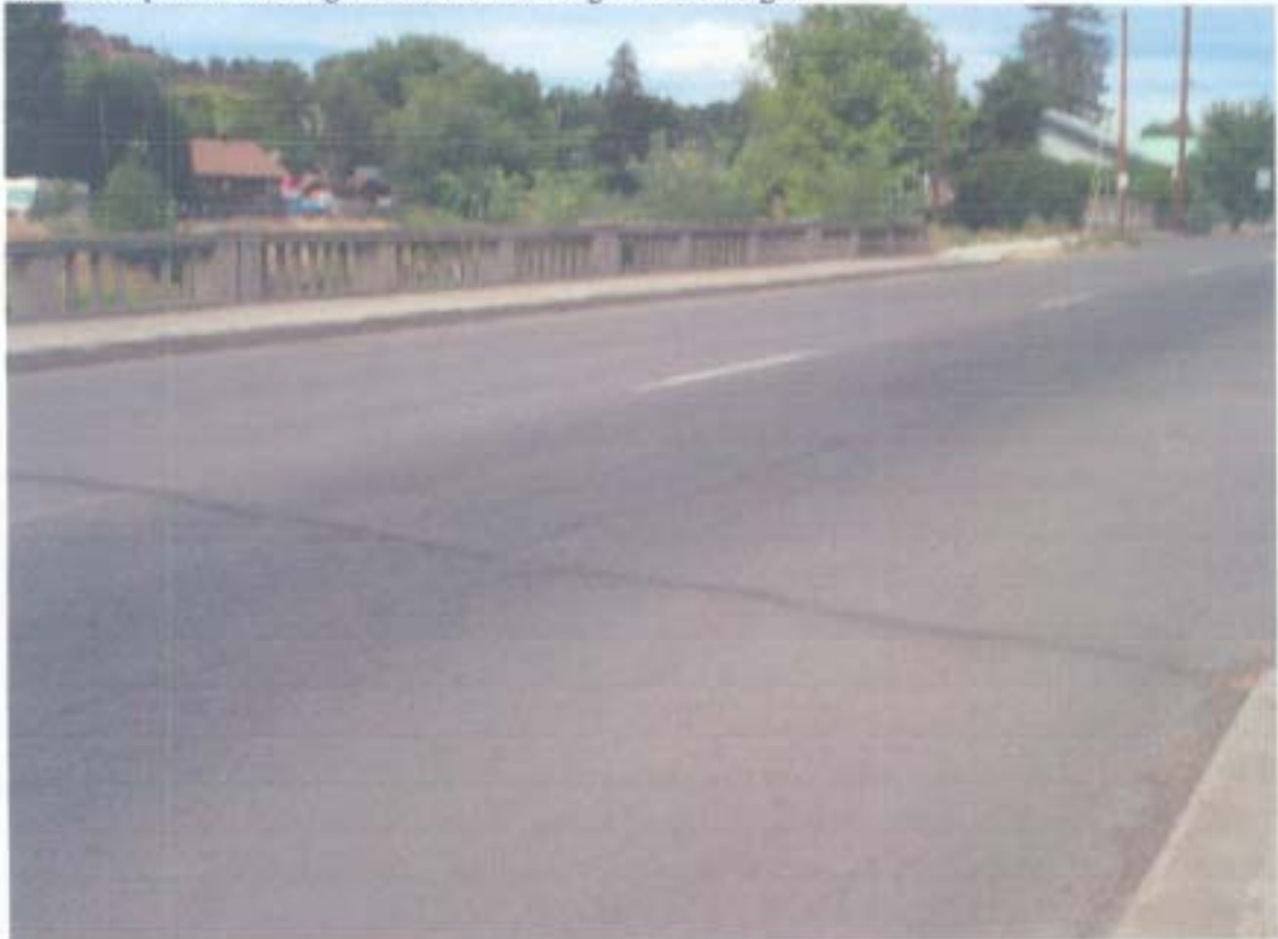
West side of bridge showing substandard and deteriorated bridge rail.
