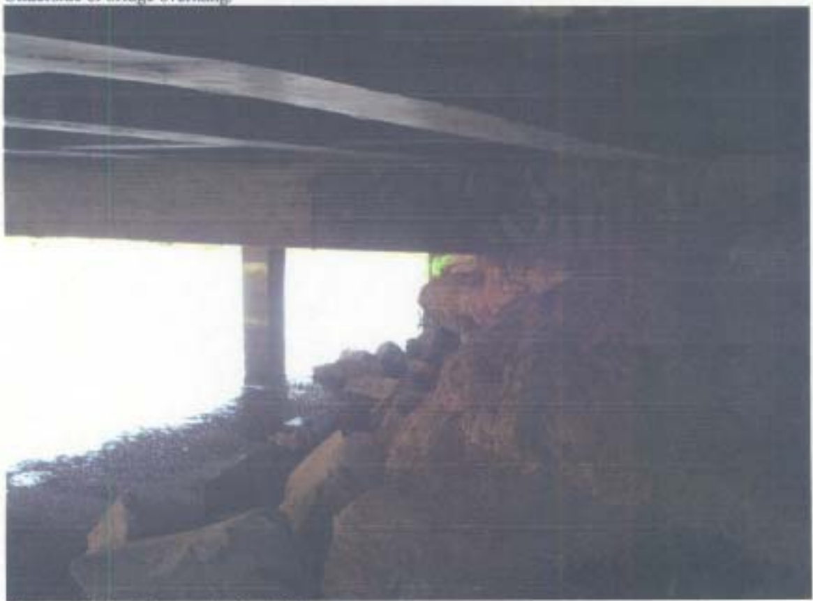
Steep eroded end slopes under the bridge.
