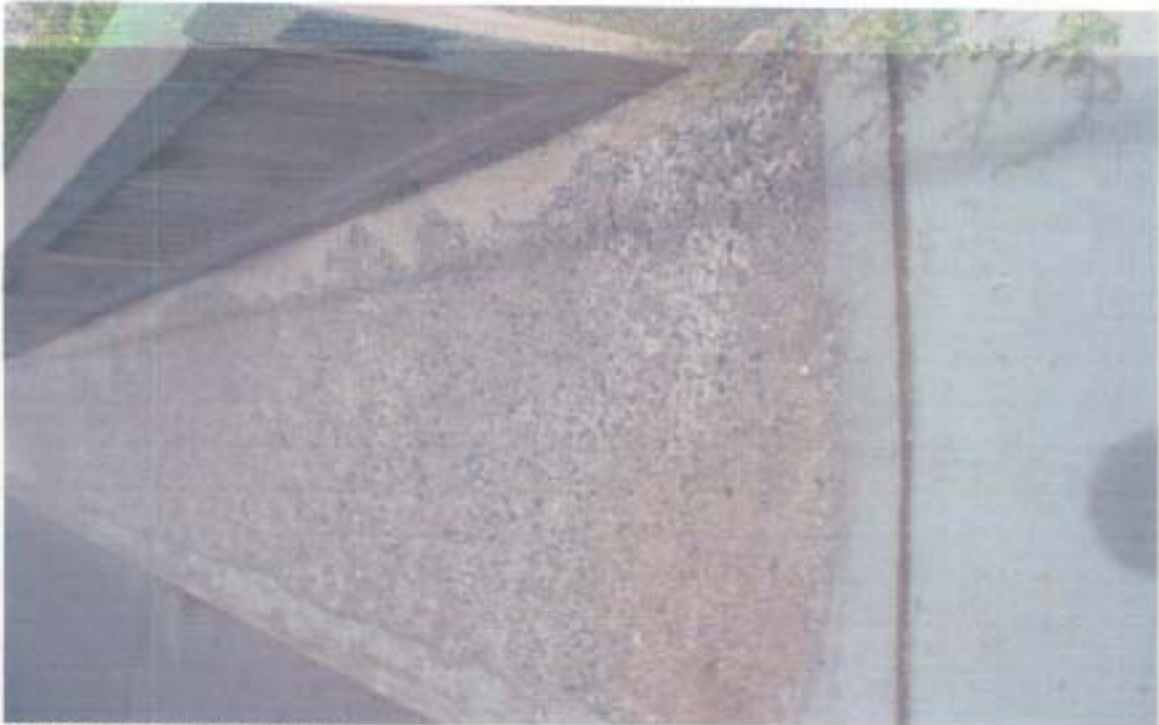
Deteriorated sidewalk on bridge.
