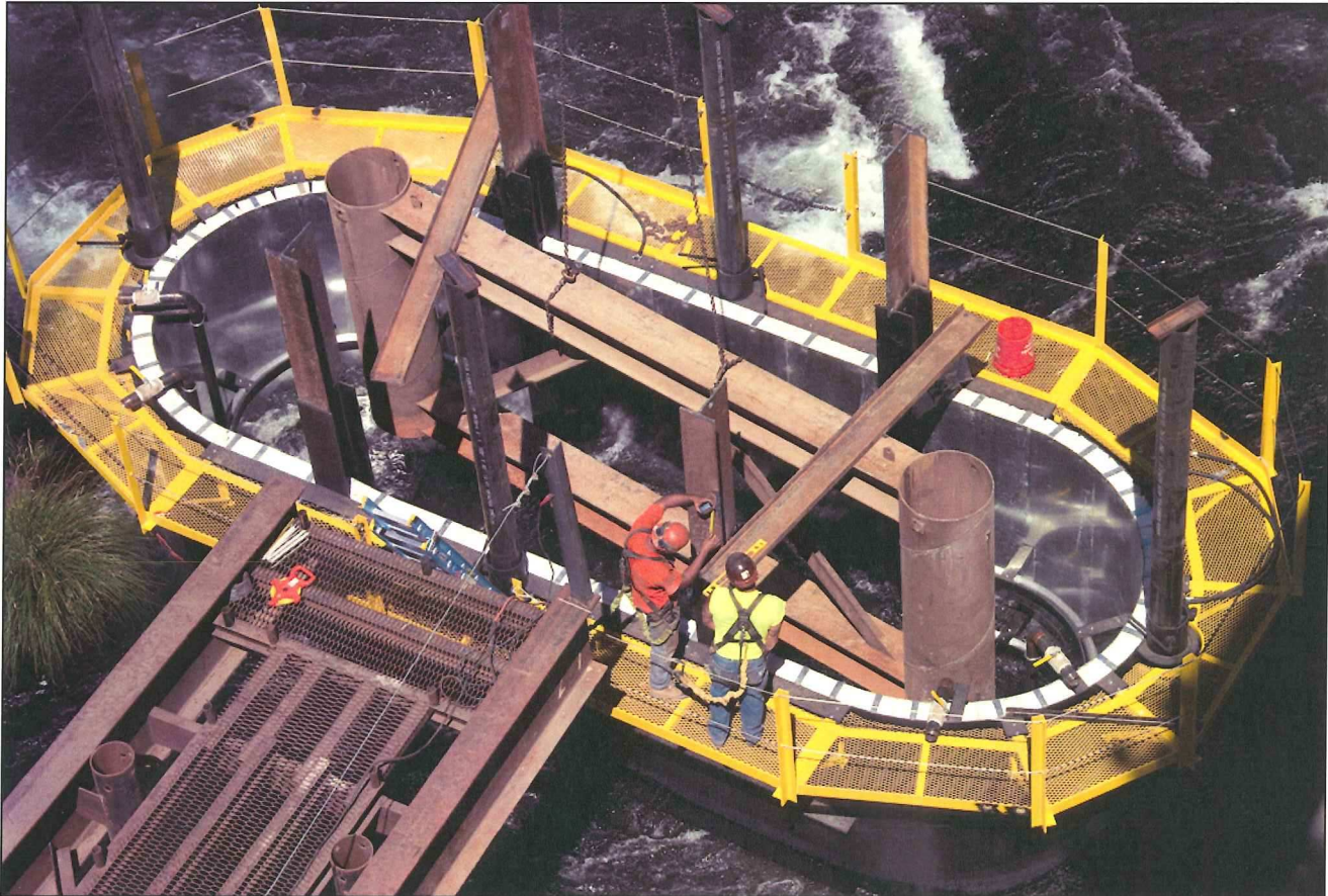
I-5: Willamette River Bridge, Bundle 220: Bubble curtain developed to meet hydro-acoustic threshold.
