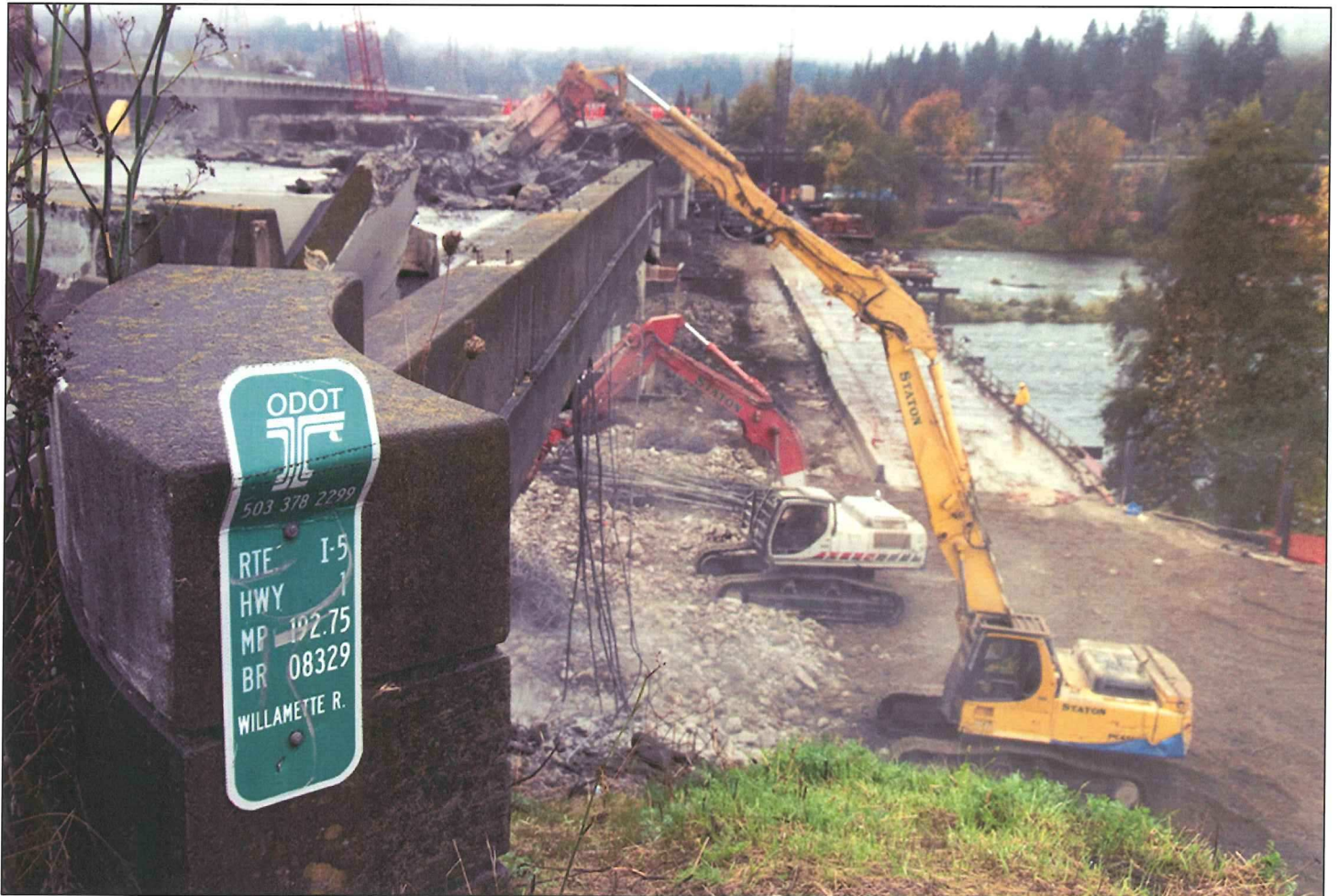
I-5: Willamette River Bridge, Bundle 220: Specially designed mechanical arms aided in a speedy demolition.
