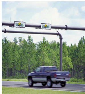
A high-speed, non-stop electronic toll portal on SR 417 near Orlando, Florida.
