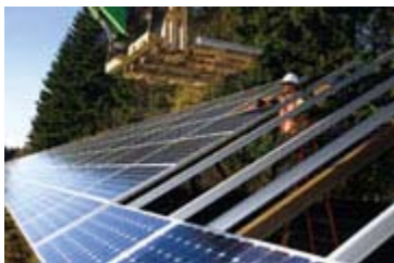
Workers install solar panels as part of the Oregon Department of Transportation Solar Highway Demonstration Project.
