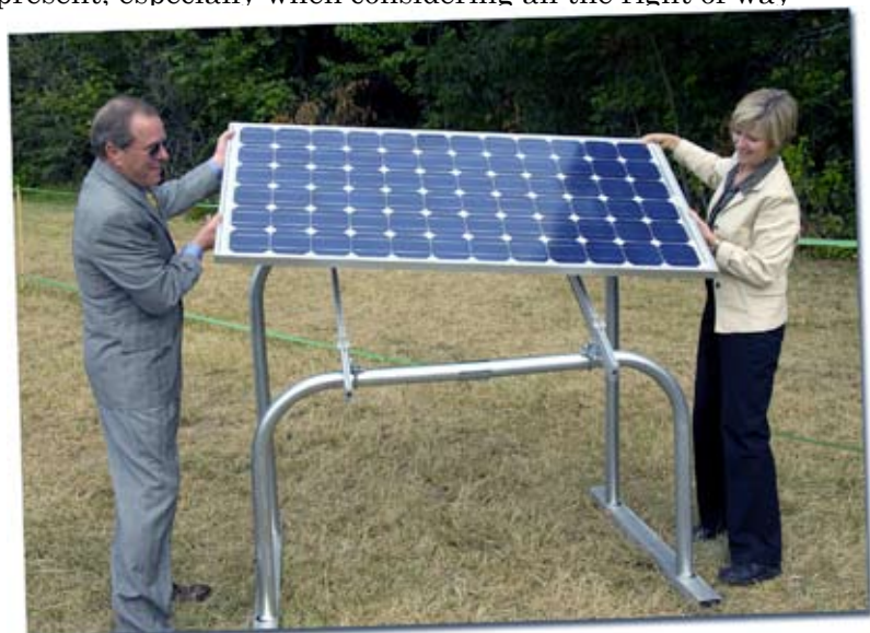
Oregon Governor Ted Kulongoski and Portland General Electric CEO Peggy Fowler install the first solar panel in Oregon's Solar Highway.
