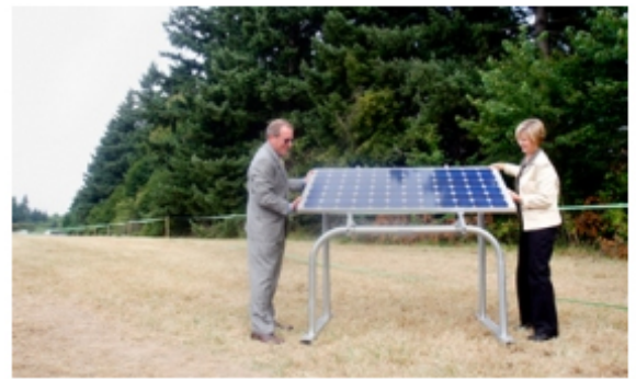
JONATHAN HOUSE / PAMPLIN MEDIA GROUP Gov. Ted Kulongoski and Portland General Electric Chief Executive Officer Peggy Fowler install the first solar panel of an array that will be used to power highway lights at the I-5/205 interchange in Tualatin.
