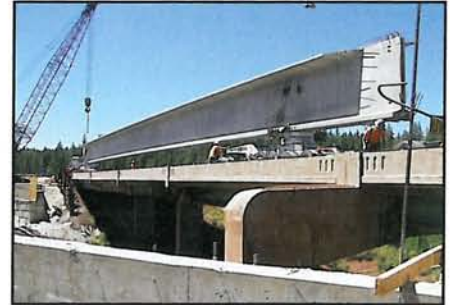
Time Saver Pre-cast single span beams (above) reduced construction time and traffic delays on U.S. 97 near Chemult, Ore. Fish Friendly Workers (below) activate a "bubble curtain" around a bridge piling to muffle construction.
