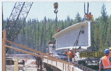
The Oregon bridge program has the work being done faster and more economically than traditional methods. PHOTO COURTESY OF ODOT
