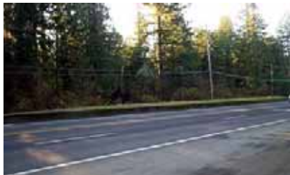
View of the concrete retaining wall on the south side of US 26.
