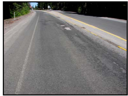
Deteriorating pavement on US 26 near Wapinitia Junction.
