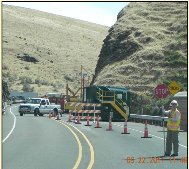
A flagger stops southbound traffic on US 97 near Biggs Junction during the Regions 4 & 5 Work Zone Safety Audits in August 2011. In addition to the evaluation scores, the Safety Audits also provide opportunities to take pictures for examples of devices in the field, examples of TCP deployment, and examples for training classes.
