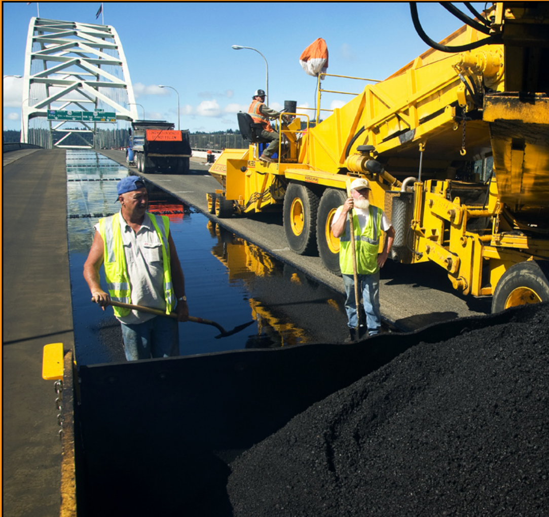
Paving crews work on the upper deck of the Fremont Bridge (Southbound Interstate 405) in Portland in July 2011. The project required three weekends of full closure of Southbound I-405, along with several weeknights with multiple lane closures. The Fremont Bridge is the only bridge in Oregon with an epoxy asphalt concrete pavement wearing surface, which requires a minimum cure time of two hours before traffic can drive on it.
