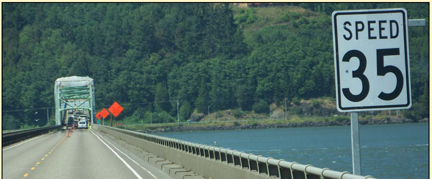
Reduced construction speed limit signing on US 101 at the Astoria-Megler Bridge near Astoria. The temporary flagger signs (left) are mounted to rotating posts that are turned away from traffic when they are not needed. The base of the rotating posts are pinned to keep the signs properly aligned in high winds near the mouth of the Columbia.
