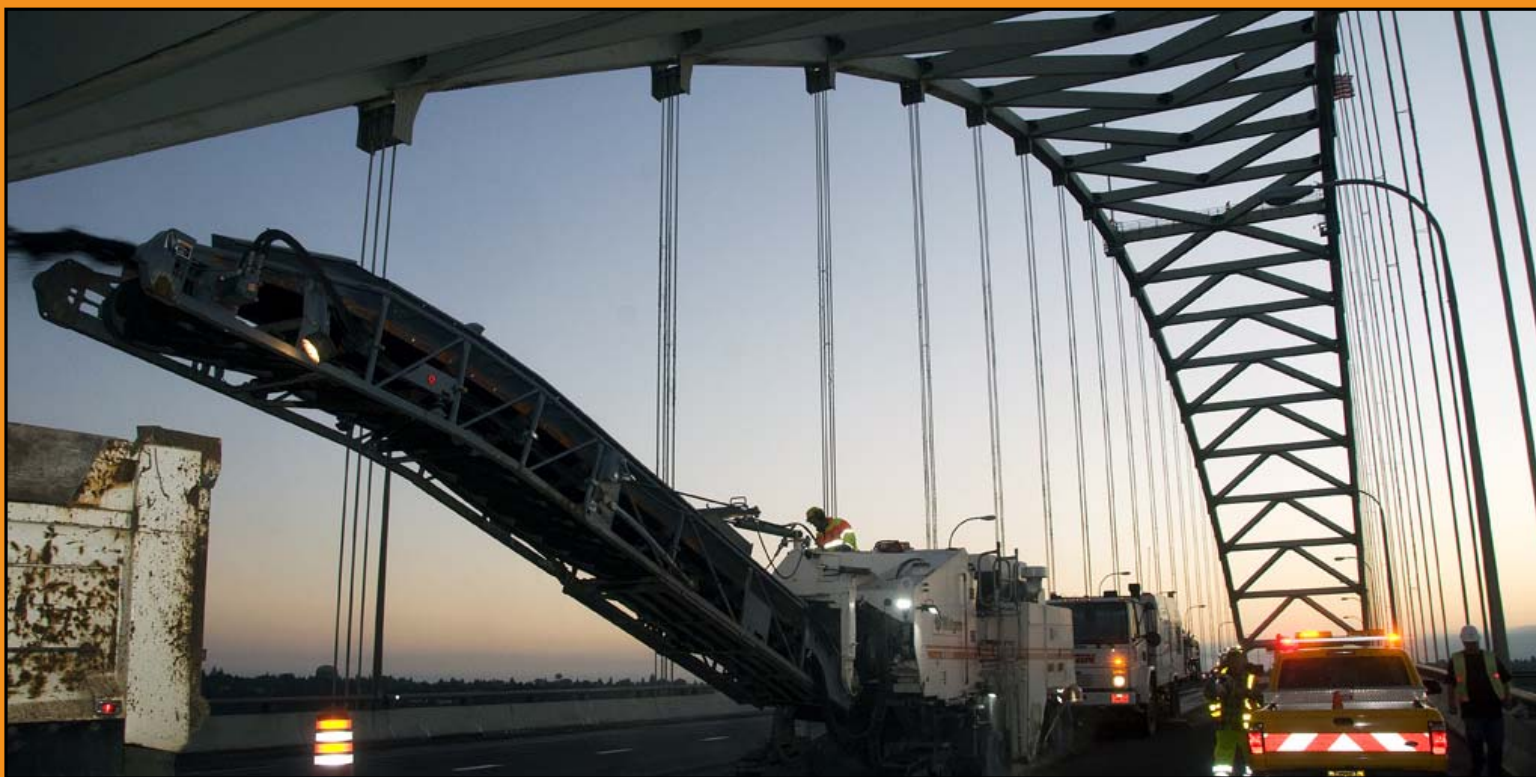
Pavement removal operation on the upper deck of the Fremont Bridge (Southbound Interstate 405) in Portland in July 2011. The paving project required three weekends of full closure of Southbound I-405, along with several weeknights with multiple lane closures. Traffic was detoured around full closures to the I-5 Marquam Bridge, south of downtown Portland.
