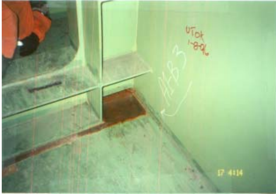
Figure 5.4: Fatigue Category E' detail found in box girders at diaphragm connection to flange. The detail does not effect the butt welds.
