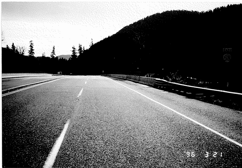
Figure 2.12: Motorist view of blockmat.
