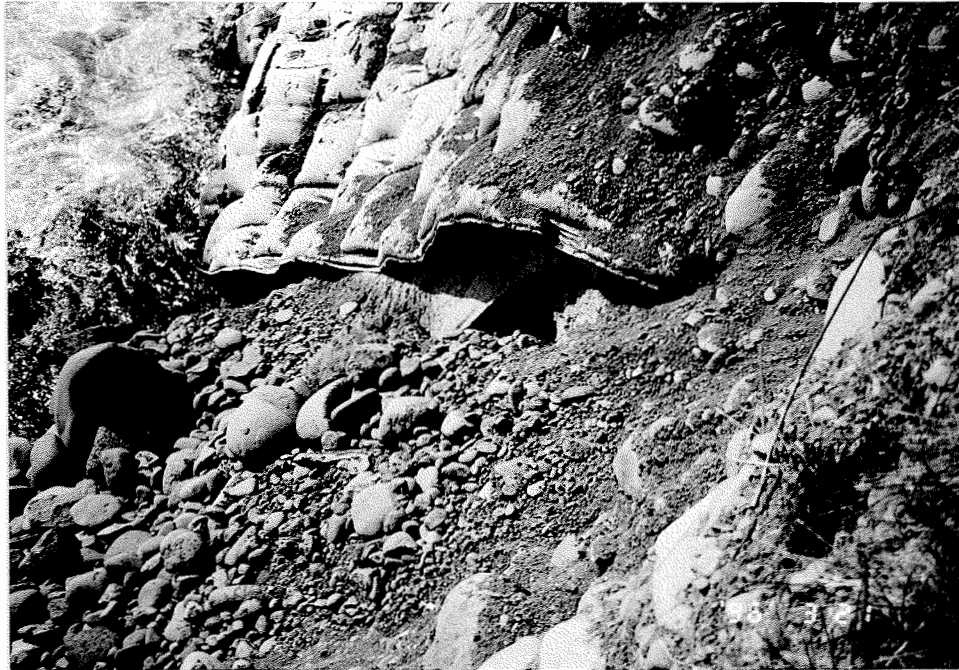
Figure 2.7: Northwest corner of ABM, note undermined edge.
