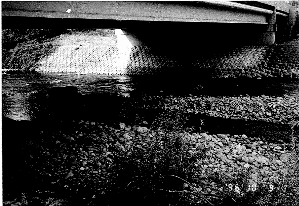
Figure 2.11: Most of the west side was not damaged.
