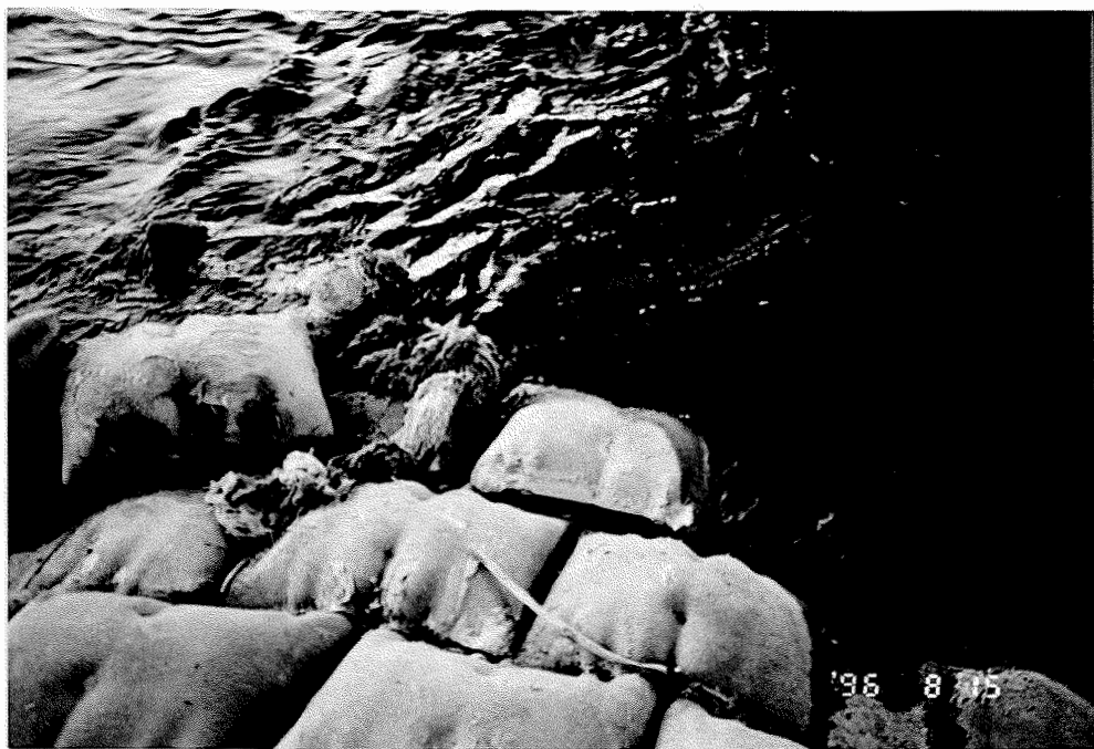
Figure 2.10: Blocks in damaged area are held only by fabric bag.
