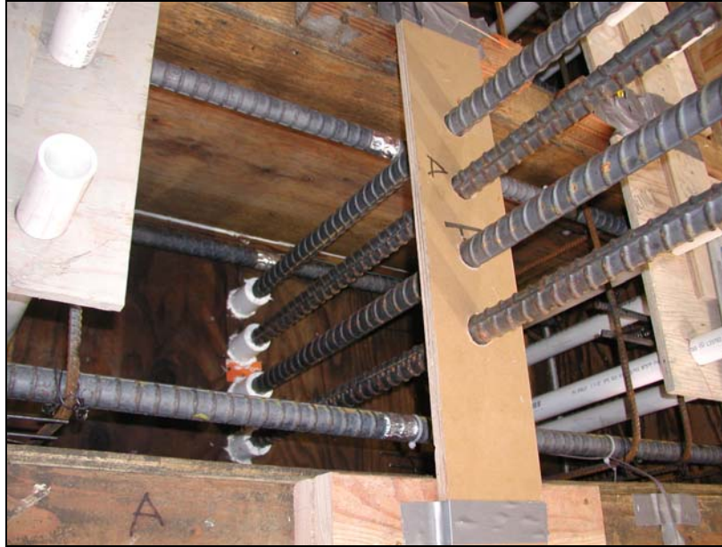
Figure 2.6: Typical low confinement column cage prior to casting (no ties located in the anchorage zone)
