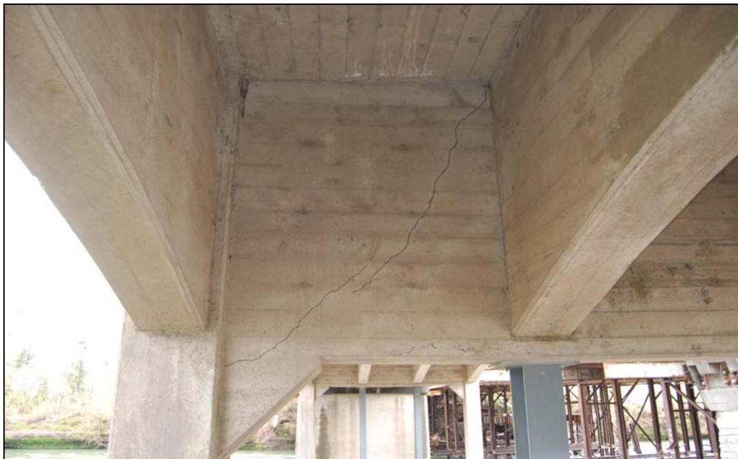
Figure 2.1: Typical diagonal crack forming at column bent connection (diagonal crack highlighted)
