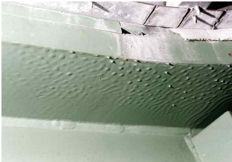
Figure 6 (71056-12) Top Flange Weld Thickness Transition; Weld Crown Ground Smooth; Weld Not Visible
