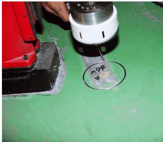
Figure 22 (71149-13) ESW weld during core drilling
