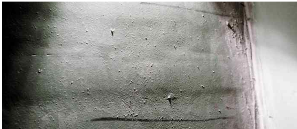
Figure 4 (71056-02) Bottom Flange Weld; As Ground During Construction
