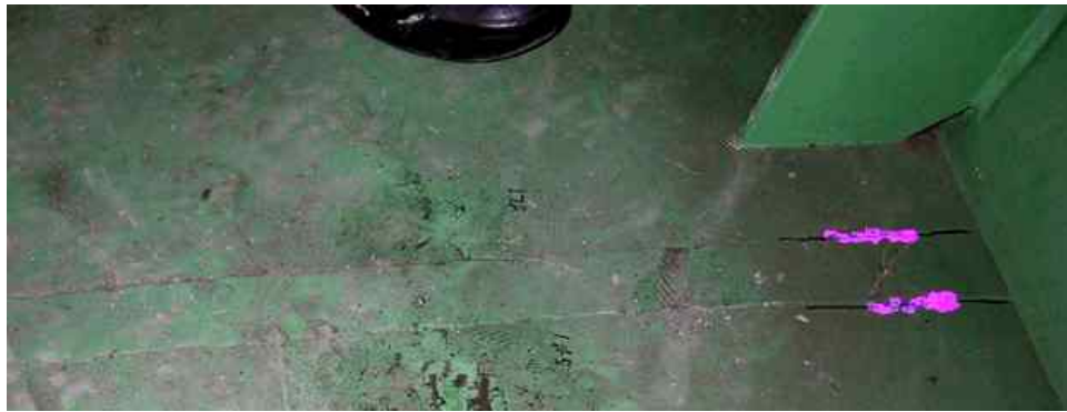
Figure 3 (D71055-08) Bottom Flange Weld
