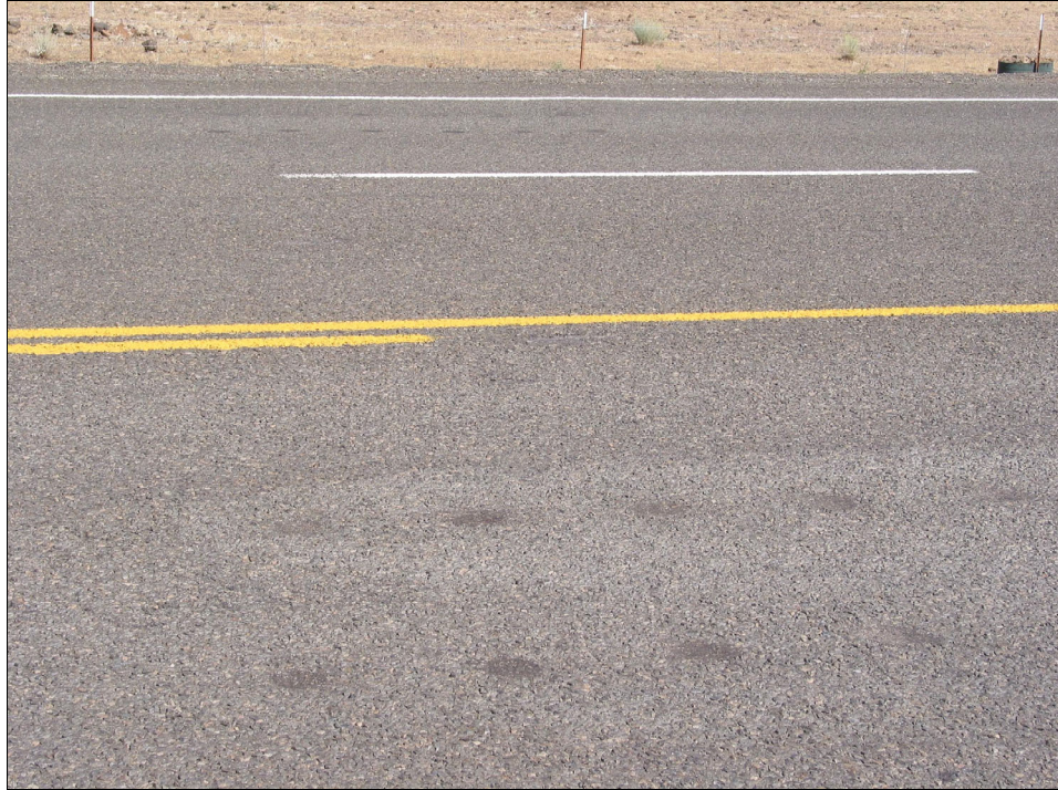
Figure 2.8: Photo of the coring locations after 14 months – solvent-free in foreground
