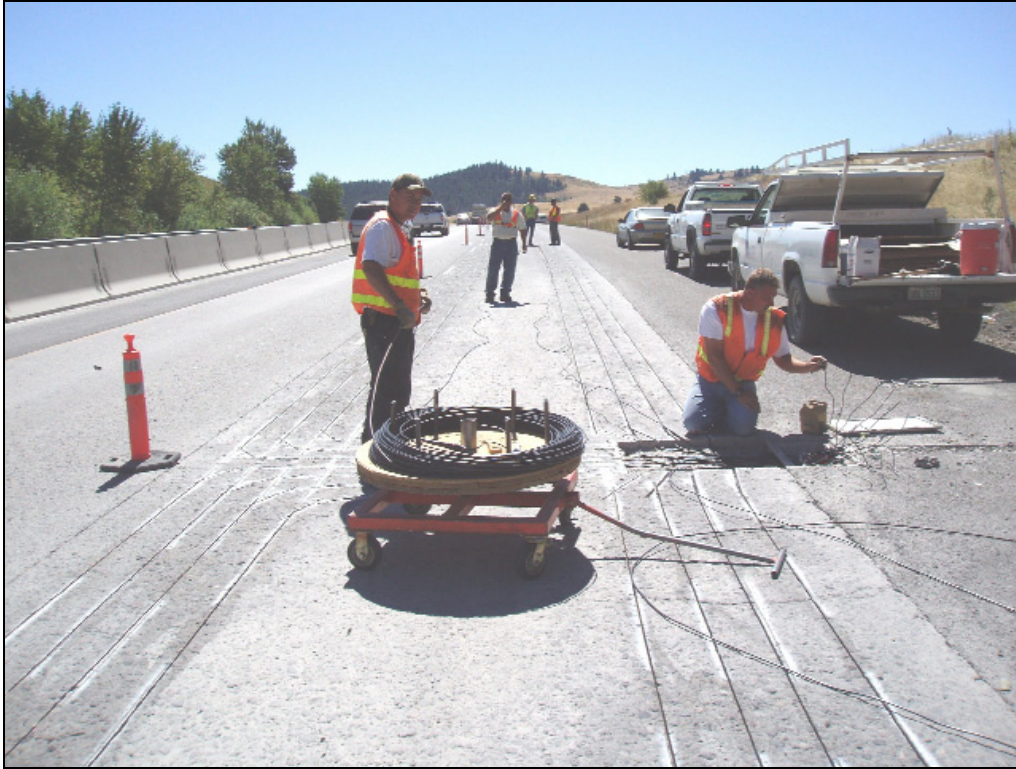
Figure 3.2: Electric heating cables in tire paths
