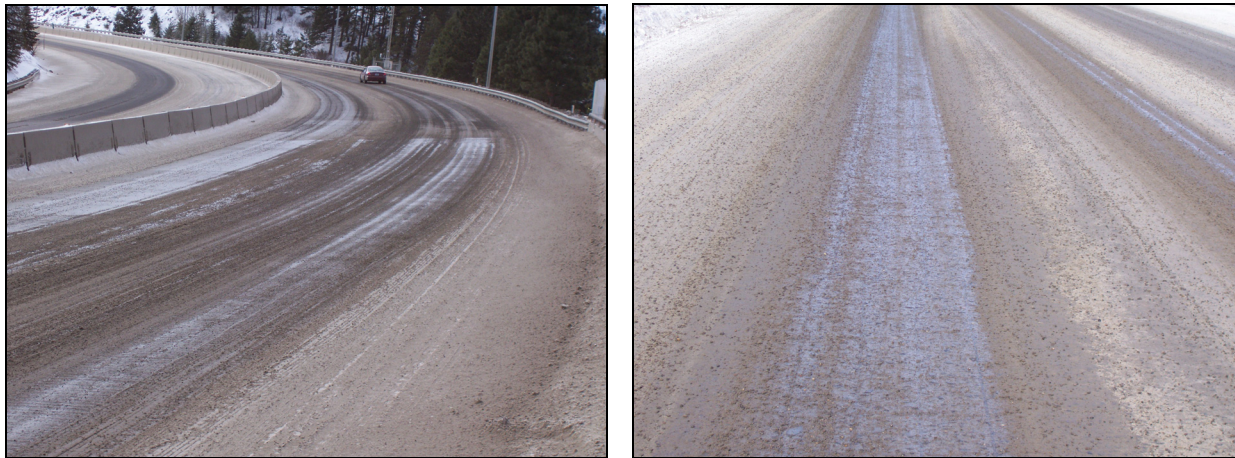
Figure 5.1: Melted snow on tire paths due to heating cables
