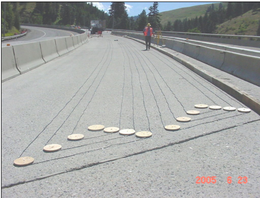
Figure 3.1: Electric heating cables on bridge deck
