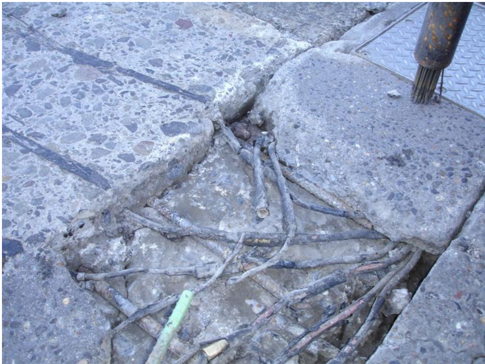
Figure 4.1: Damaged heating cables
