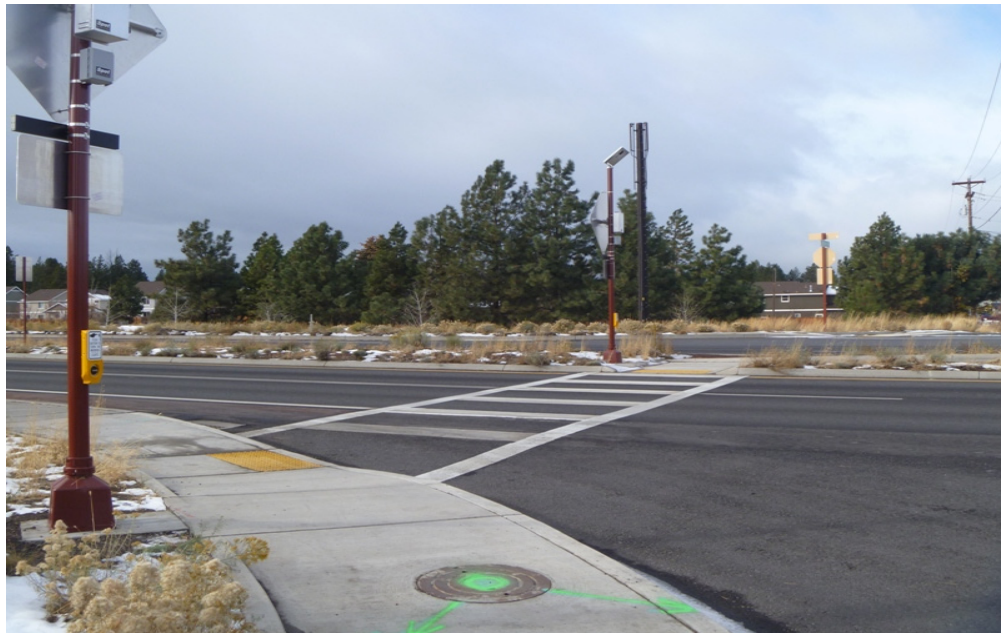
Figure 3.5 Pedestrian's perspective of RRFB installation at the Bend Parkway and Badger Road
