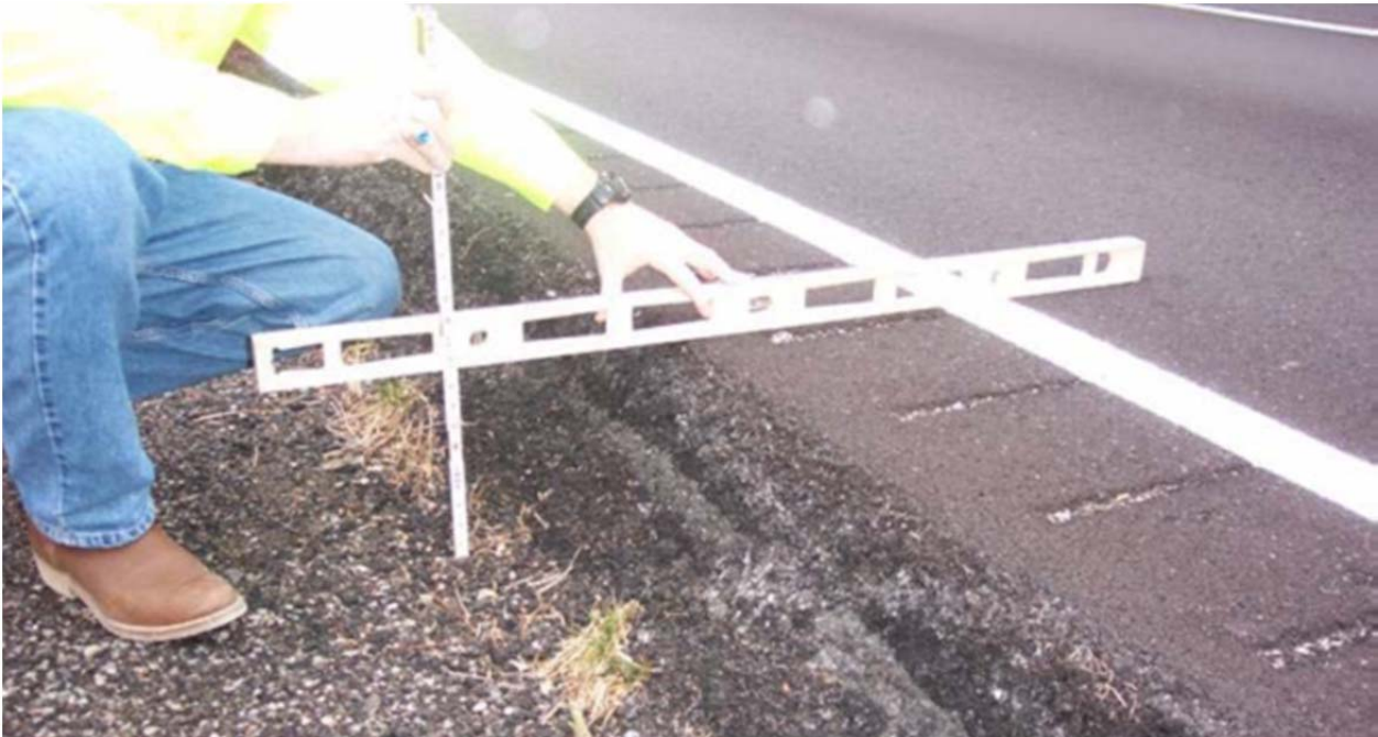
Figure 2.6: Example of Pavement Edge Drop (Kirk 2008)
