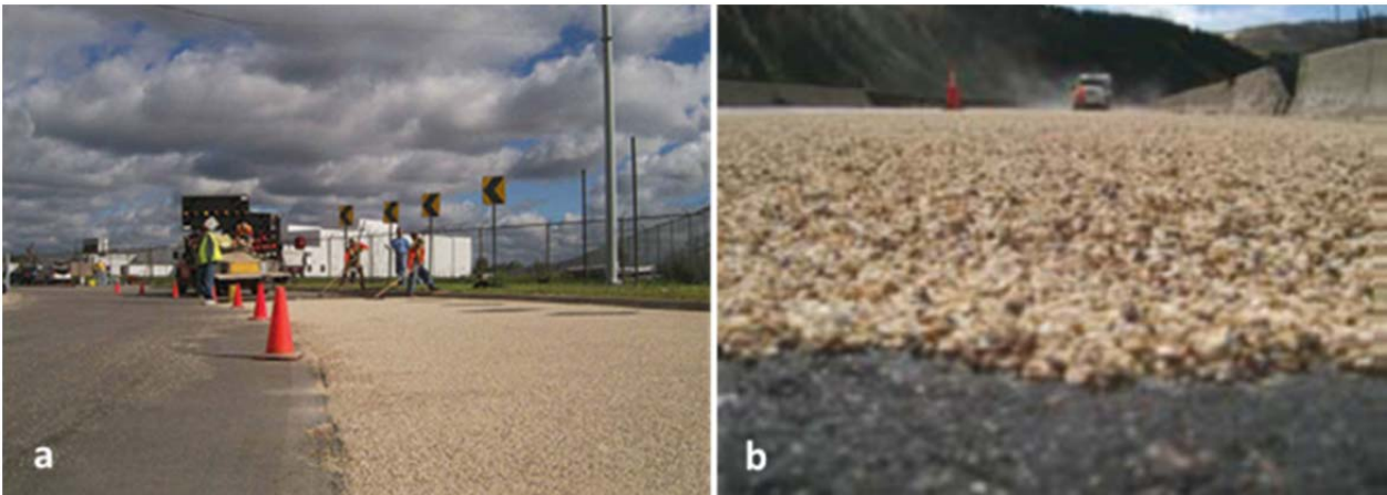
Figure 2.4: Pavement Friction Improvement Measures (a – ( Veneziano and Villwock-Witte 2013 ), b – ( Veneziano et al. 2011 ))
