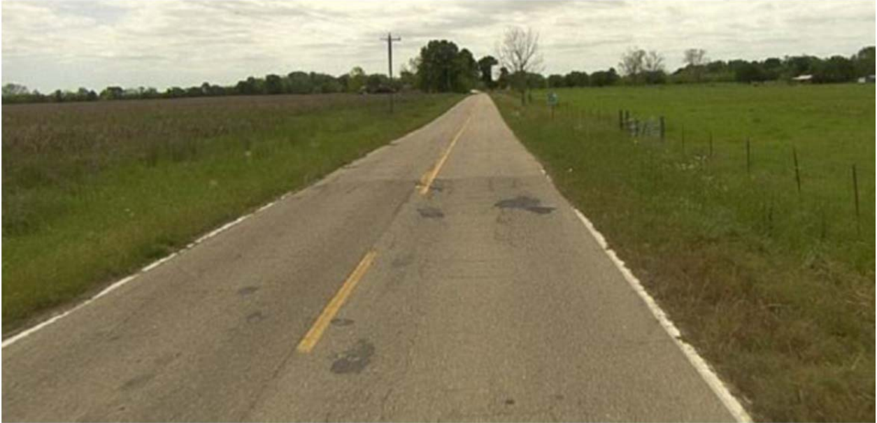
Figure 2.5: Example of Road that may Benefit from Shoulder Improvements ( Sun and Das 2012 )
