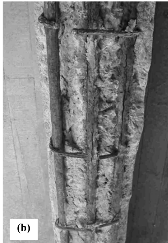
Figure 1.5: Broken shear stirrups along base of reinforced concrete deck girders on the Spencer Creek Bridge: (a) south span; (b) north span. There were no broken shear stirrups in the central span.
