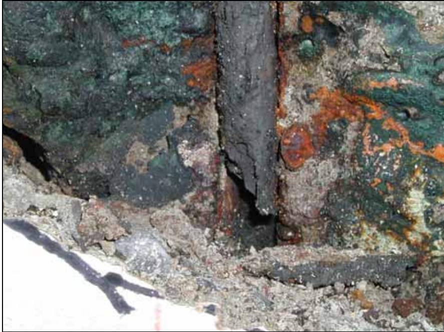
Figure 4.3: Completely corroded shear stirrup in bottom third of beam where shear crack formed
