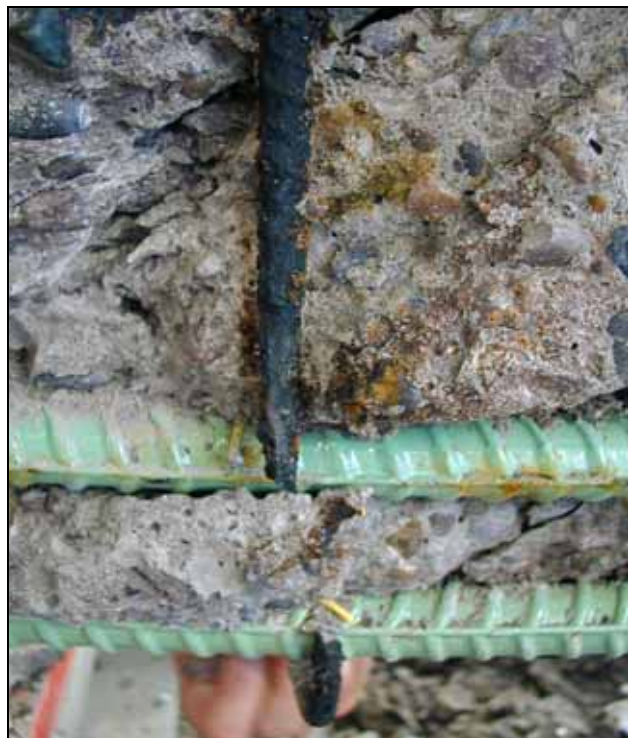
Figure 4.4: Fractured shear stirrup near flexural tension steel
