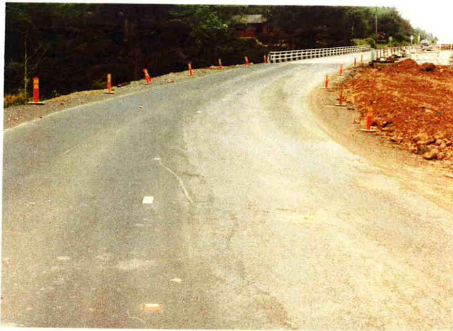
6/10/77 Southbound view from near sta. 1872. Note nailed reflector in foreground and use of reflective tape.
