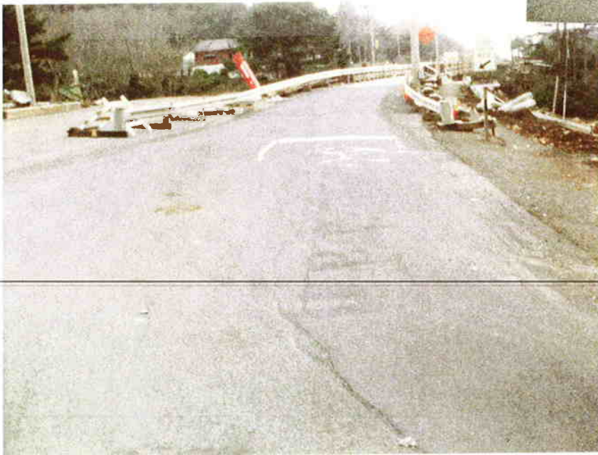
3/22/77 Temporary stripe to identify lanes more clearly at north traffic signal stop line near sta. 1872.
