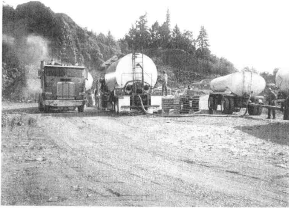
a) Equipment near blending unit. From left to right: transfer truck, blending unit, and tanker with base asphalt.
