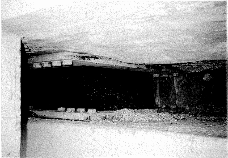
Figure 4.1 The bearing at bent 7 of BR.# 9669A is inclined to vertical and has rust on the steel plate.
