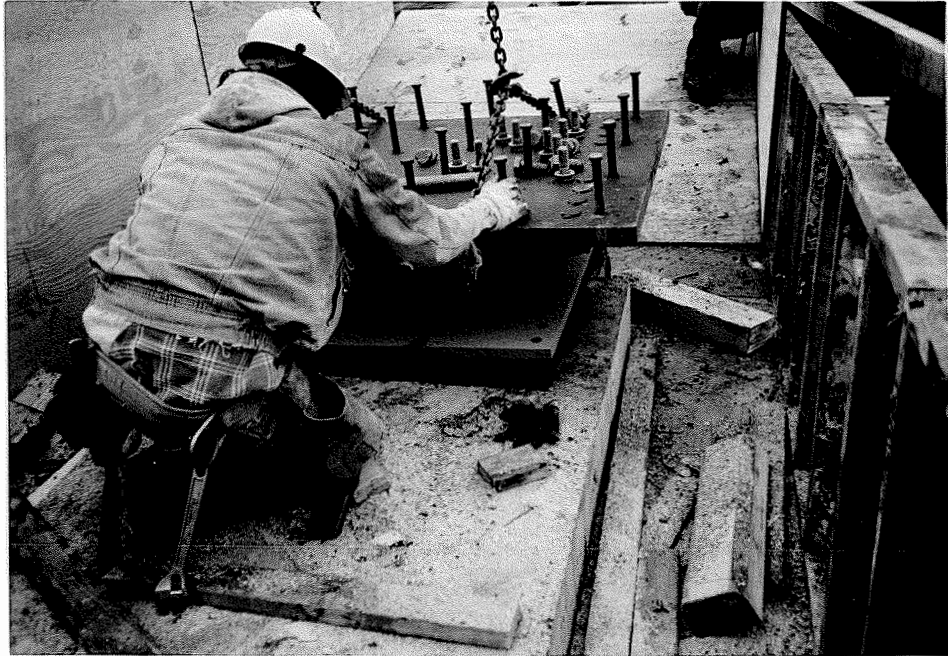
Figure 3.1. A worker prepares the isolation bearing to be lifted to the top of a column of BR# 9669A. Note the shear pins at the top of the steel plates.
