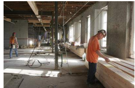
Kobbi R. Blair | Statesman Journal Restoration work continues Thursday on the third floor of the 126-year-old J Building of the Oregon State Hospital building.
